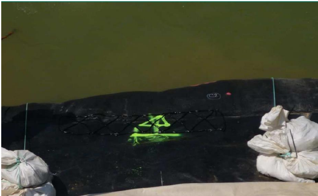
Figura3: Axis of the defect marked on the Berm
