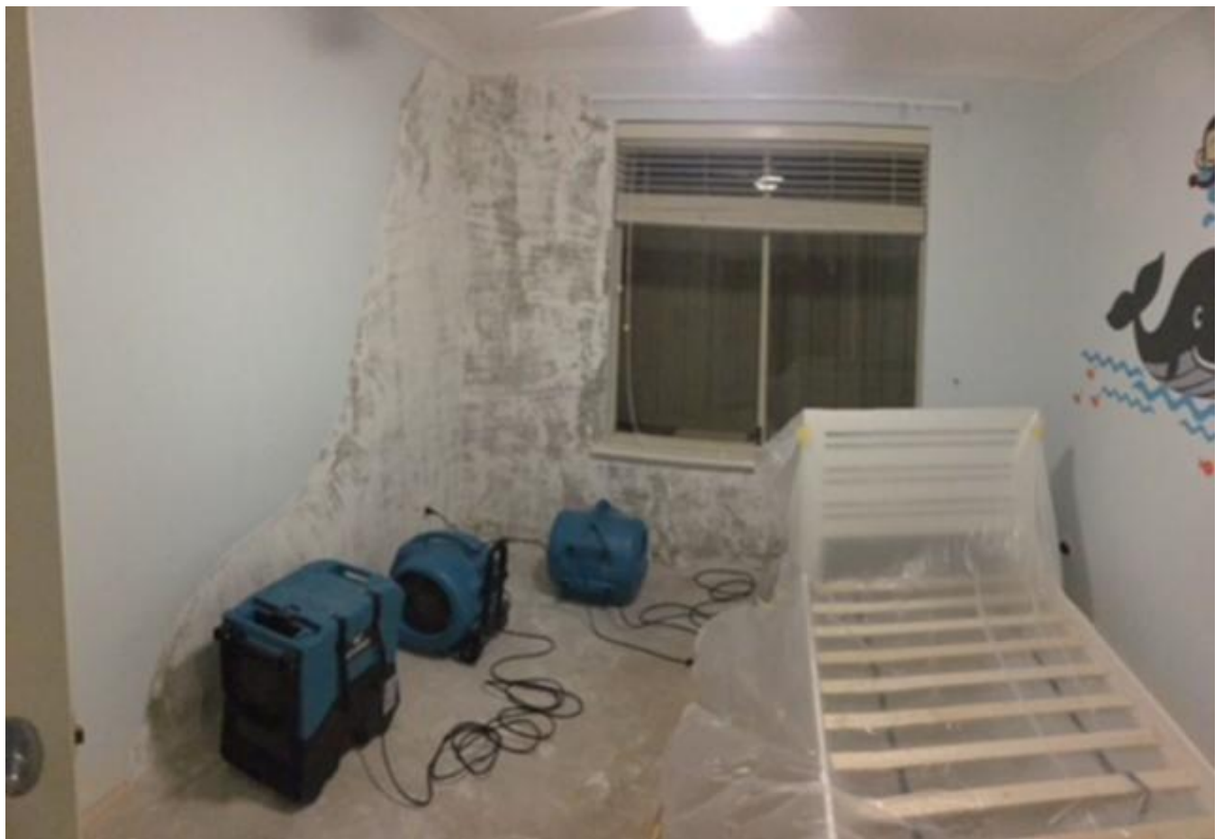
📷 Dehumidifiers in action in the waterlogged Jane Brook home of Damon Connaughton. The house was flooded several times due to defective Iplex piping. Credit: Supplied
