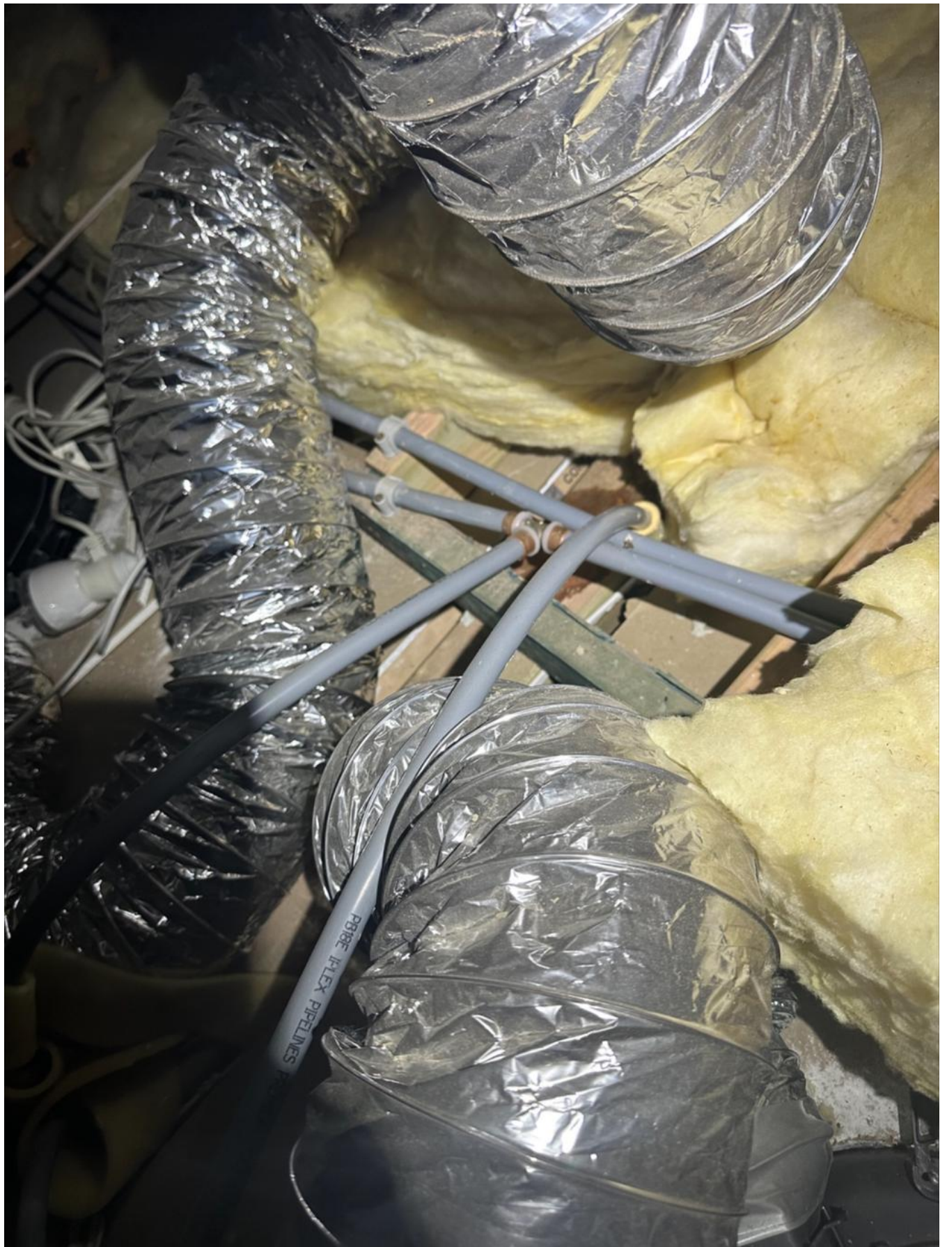
📷 Manufacturing defects in Pro-fit polybutylene pipes made by Iplex Australia and installed by BCG and Delstrat Groups. Credit: Supplied
