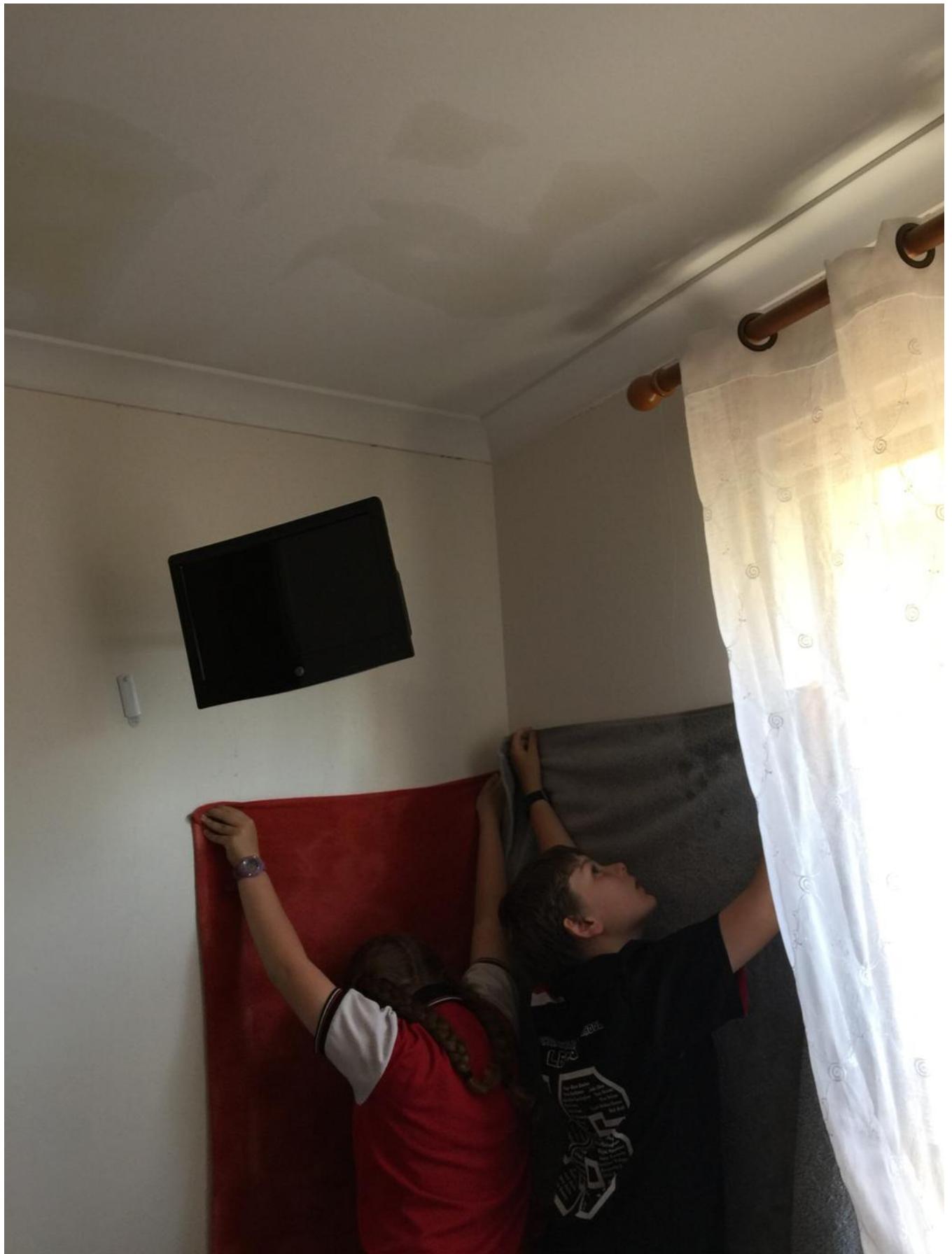
📷 Thomas and Tahlia Stokes holding towels below a leak in their family home. Credit: Supplied
