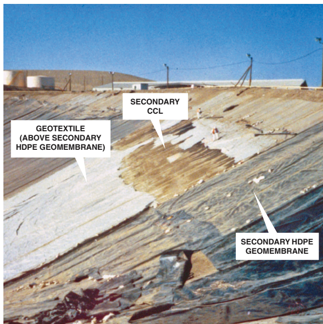
Fig. 5. (Color) Tear in geotextile layer (shown) and underlying secondary HDPE geomembrane above secondary CCL along northwest slope. (Reproduced from Byrne et al. 1992, © ASCE.)
