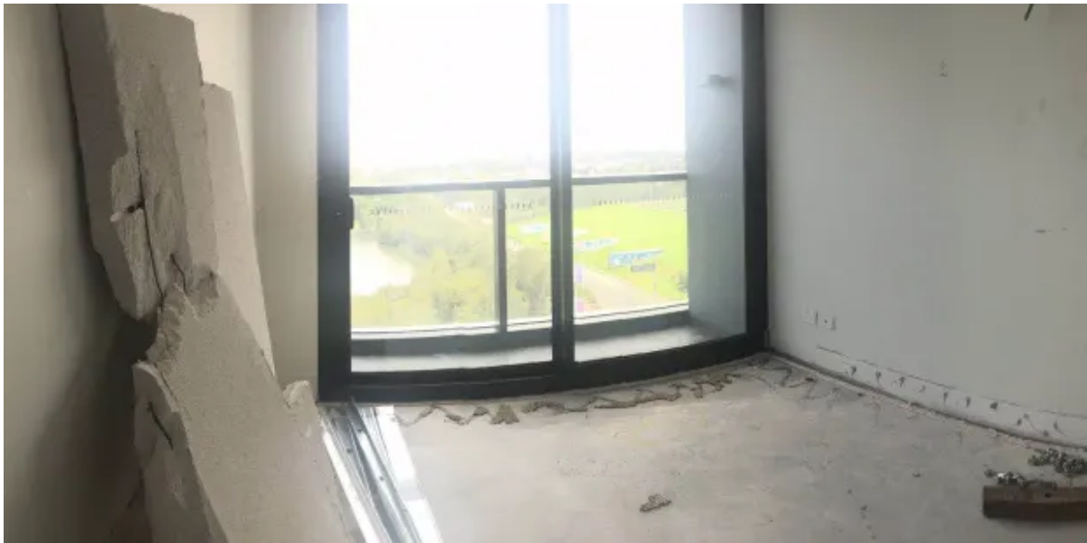
Damage to apartments in Opal Tower, showing props holding up various parts of the building, walls being cut out and major cracking. Supplied
