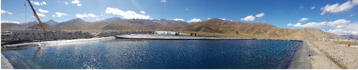
Image: In Langkazi, Tibet a 15,000 m 3 PTES with a capacity of 700 MWh of heat was constructed and professionally sealed by Solmax.
