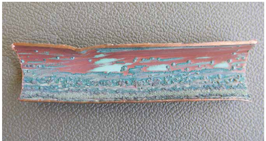
If PPR pipe fails, it generally occurs in the same location within the building, depending on which multiple simultaneous factors it was exposed to. In my experience it is typically a very small percentage of the total amount of pipe that is affected. This image is of a transition between a totally oxidised pipe to further down the line where the majority of the pipe was undamaged. Different factors are more prevalent in different parts of the system. The key is knowing how to turn them off.
