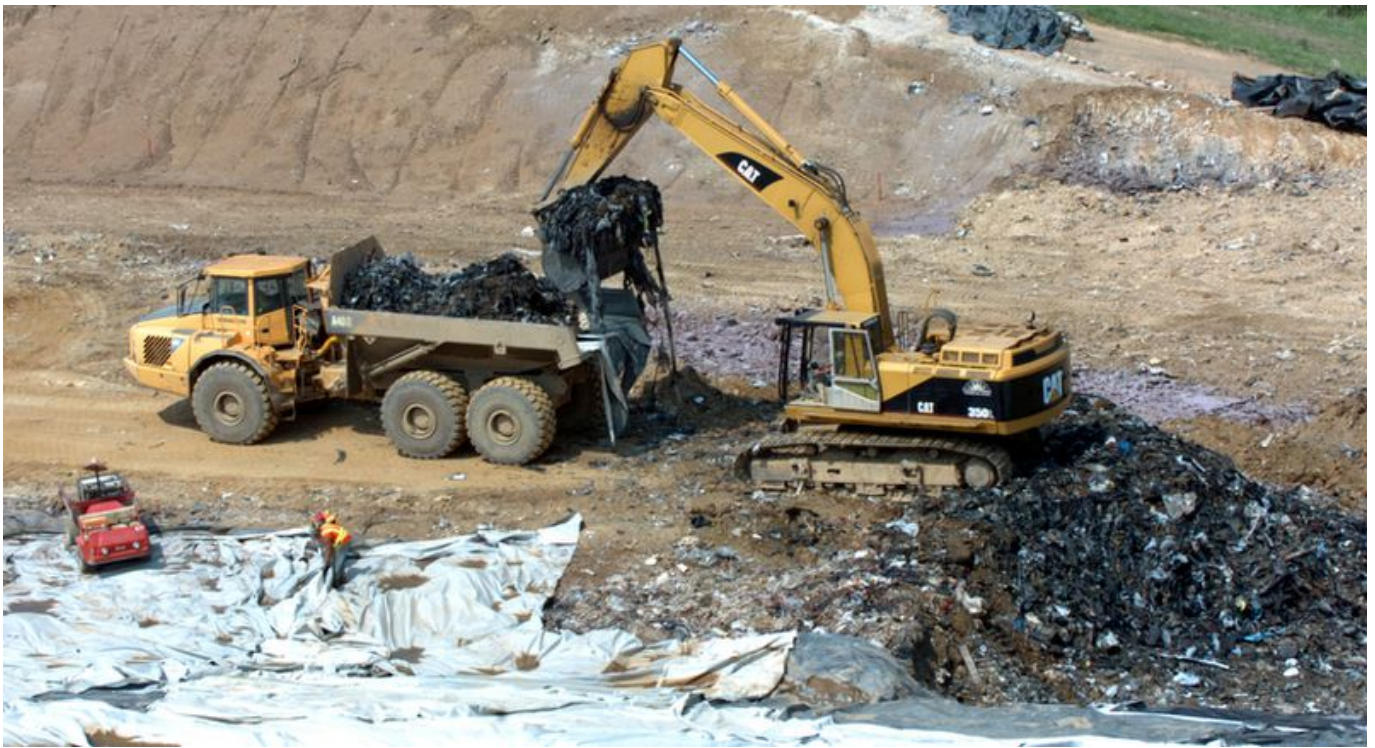
A trackhoe removes garbage on July 19, 2013, as a cleanup continues from a landslide at the Chrin Brothers Sanitary Landfill in Williams Township Express-Times file photo | Corinne Heft
