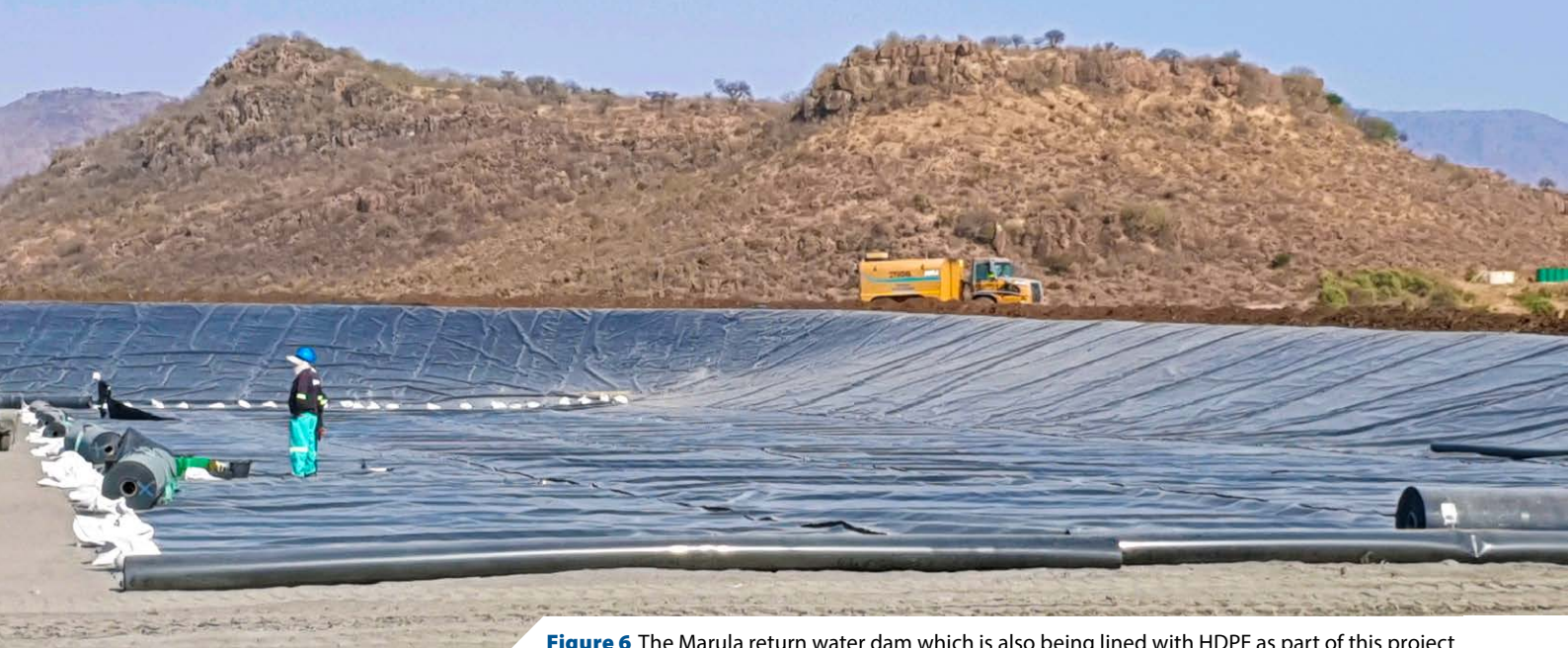
Figure 6 The Marula return water dam which is also being lined with HDPE as part of this project
