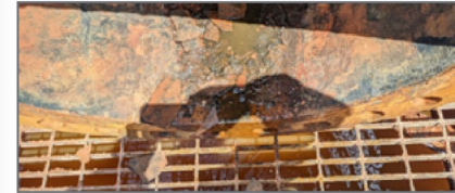
Figure 4: Scaling at 6 o'clock position
