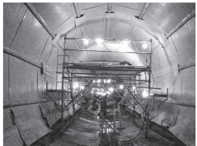
Figure 18.17 Stretching of the composite geomembrane through tightening of the external tensioning profile
