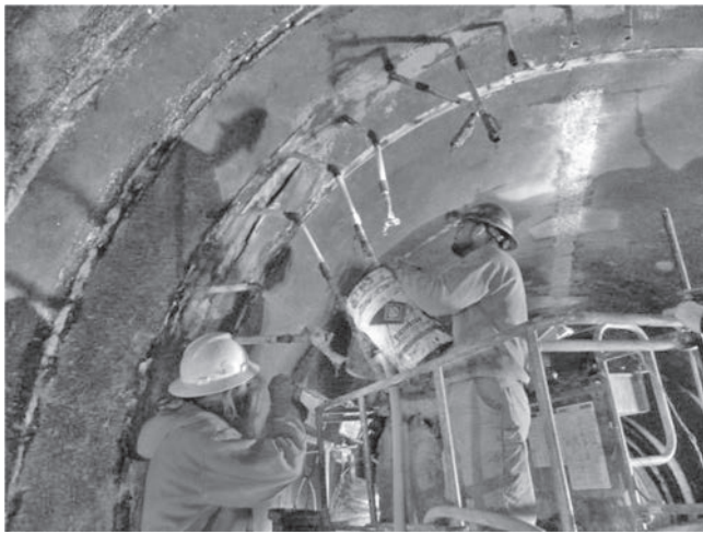
Figure 18.7 Large cracks injected with acrylic resins or cementitious grout prior to the installation of the waterproofing composite geomembrane system
