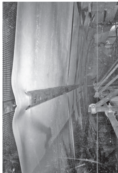
Figure 18.16 External tensioning profiles installed over a composite geomembrane to remove any slack in a pressure tunnel in Greece
