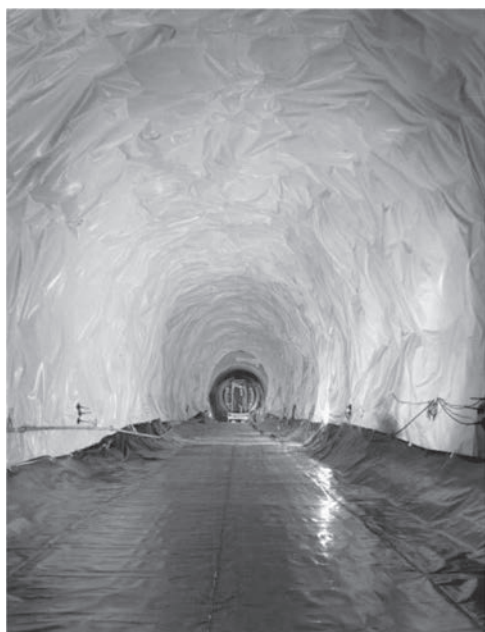
Figure 18.22 Geomembrane installed in the crown, walls and invert, and a protective sacrificial layer of geomembrane (black) in the invert
