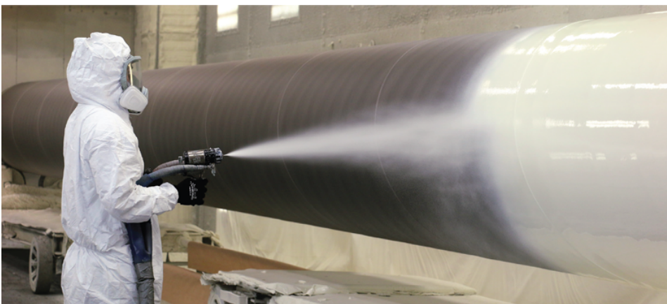
Fig. 2: Applicators sprayed a quick-setting polyurethane coating direct to metal at a minimum DFT of 25 mils on the pipe exteriors. Following inspections, they could respray any repair areas right on the line due to the coating's two-hour recoat window.
