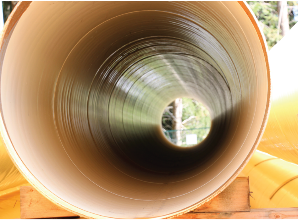
Fig. 6: The interior epoxy lining will protect the pipeline interior from corrosion and minimize the growth of microbial bacteria to maintain drinking water quality.
