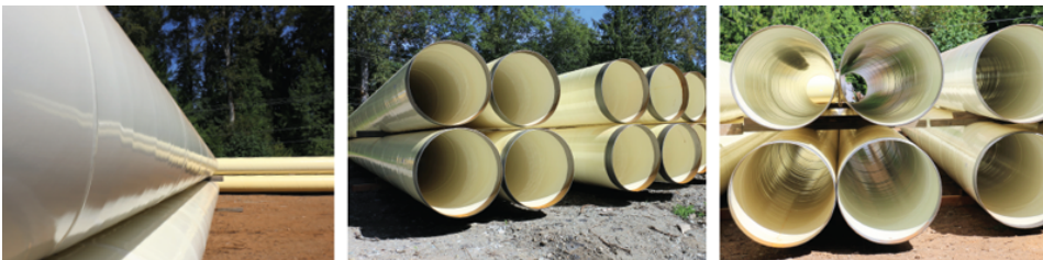
Fig. 5a-c: Fully lined and coated pipes await installation at the pipeline construction site. The coatings will protect the pipes from corrosion—inside and out.
