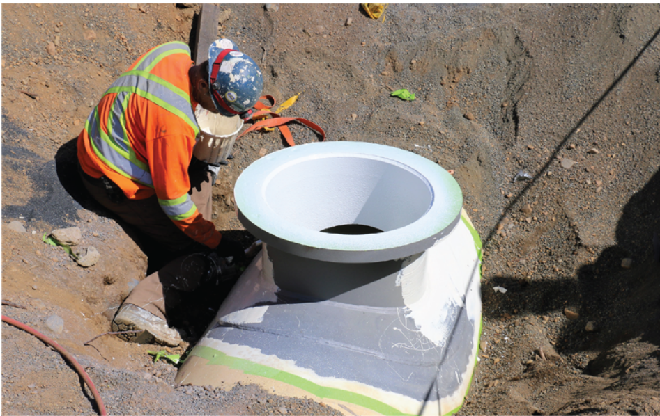
Fig. 9: An applicator brushes a quick-set polyurethane on the exterior of a pipeline access manway that was added in the field.
