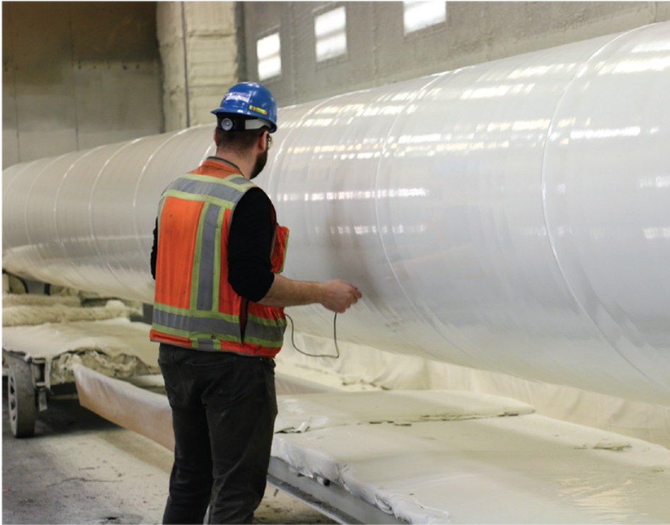
Fig. 3: Inspectors were able to begin holiday testing and DFT checks minutes after applicators sprayed the polyurethane on the pipe exteriors.
