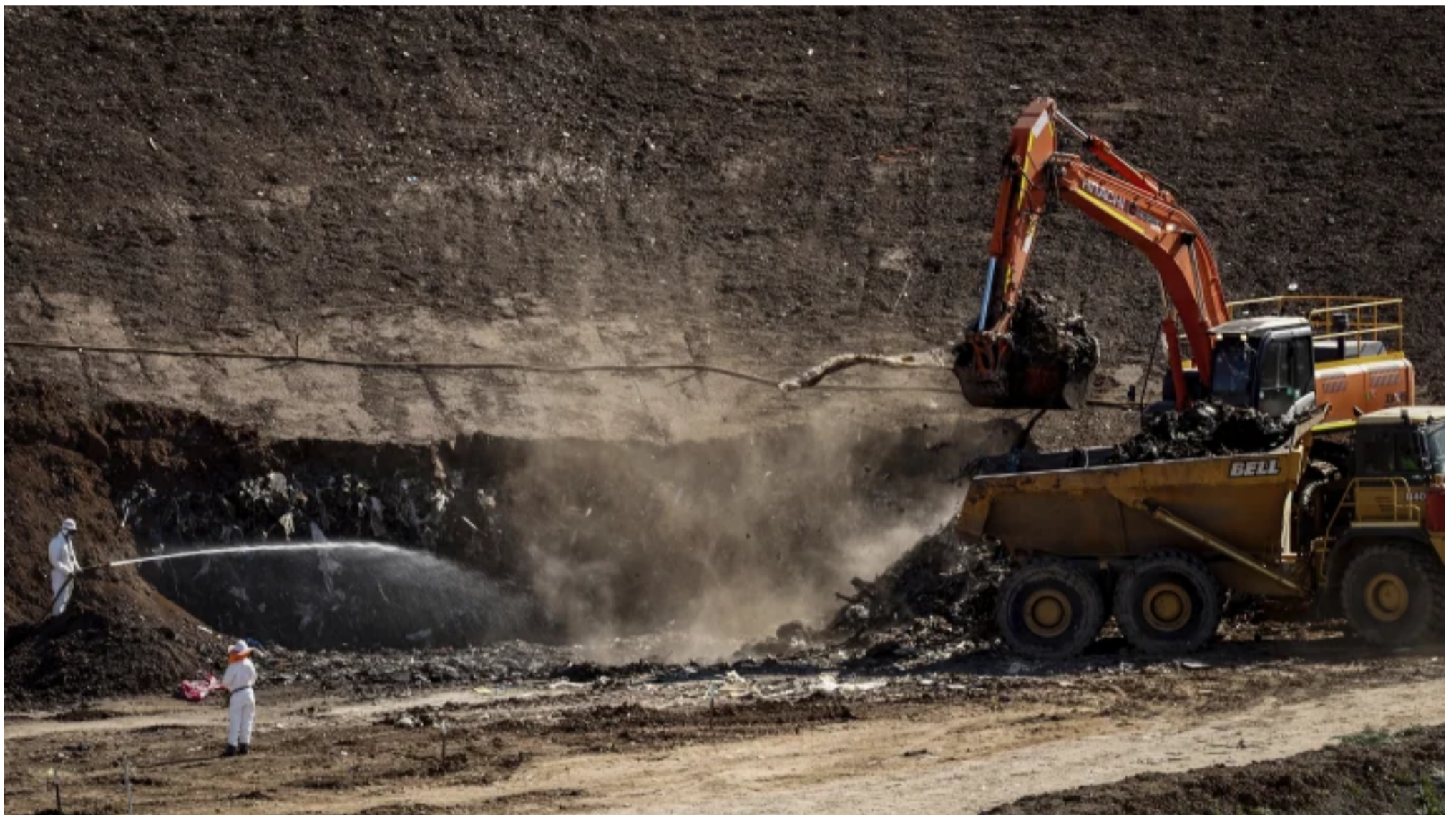
Crews working on the smouldering landfill in September last year. DARRIAN TRAYNOR
