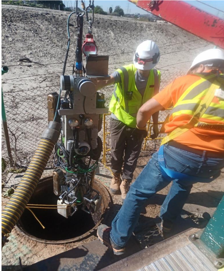
Figure 4. Workstation setup at MH H703.
