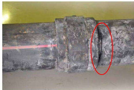
Figure 8—Pipe rupture near coupler welding joint
