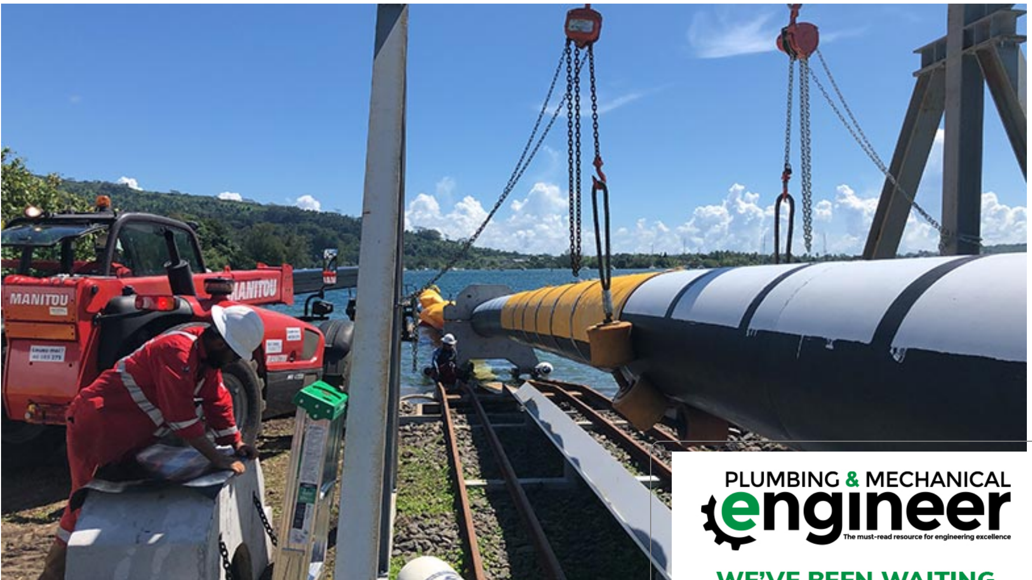
Sea water air conditioning systems provide cost savings and a reduction of greenhouse gases.
