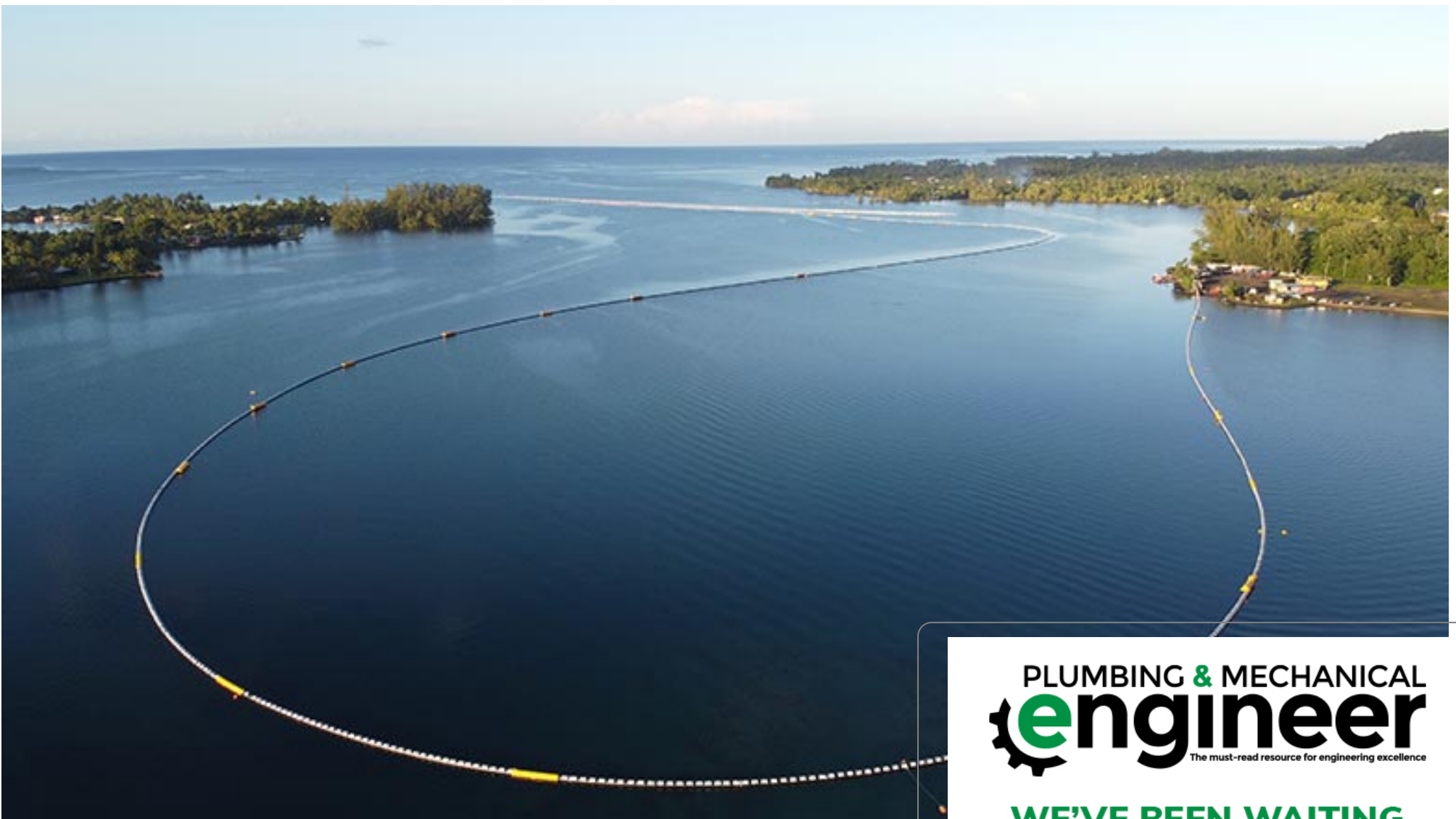
A 3,800 meter intake pipe reaches a maximum depth of 900 meters in the South Pacific.
