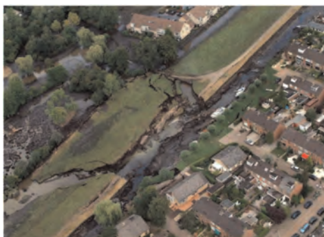
Figure 3. Aerial picture peat levee collapse, caused by dehydration during extreme draught, 2003 Wilnis Netherlands.
