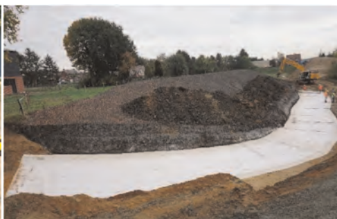
Figure 12. Horizontal installed Geosynthetic Clay Liner (GCL) in the levee foreland to enlarge the seepage length from the flood defense base.
