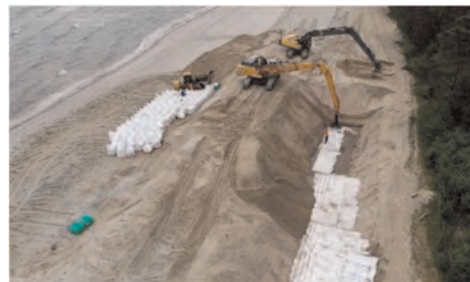
Figure 14. Installation of Geotextile Sand Containers as coastal protection measure in the dune core of the sandy beach, Ludmin Germany.
