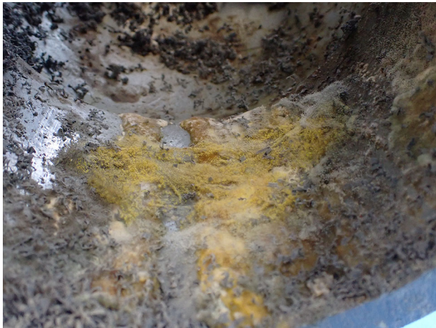
Fig. 2 Mold formation on the inner surface of the pipe-and-elbow assembly
