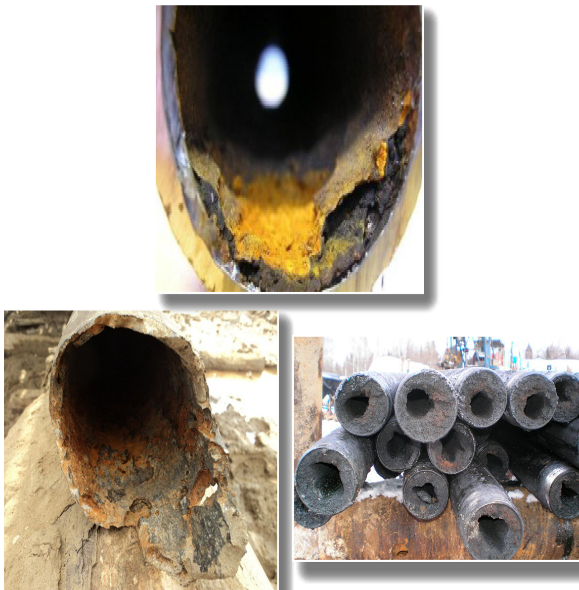
Fig. 8 Examples of corrosion caused by hydrogen sulfide.
