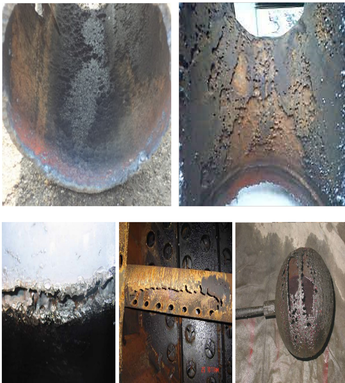
Fig. 7 Some failure parts caused by naphthenic acid corrosion (NA) [33,39].
