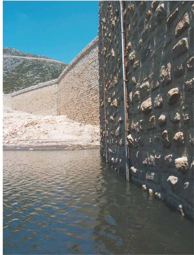
Figure 2 - Face of a masonry dam on which a nonwoven geotextile with a mass per unit area of 2000 \text{ g/m}^2 was placed prior to installing a geomembrane, Covão do Ferro Dam, Portugal [Courtesy Carpi].
