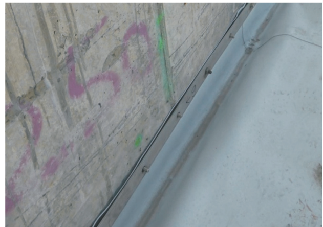
Figure 8 - Slack in the geomembrane next to a rigid structure in the Water Saving Basins of the Panama Canal Locks, 2016 [Courtesy Carpi].
