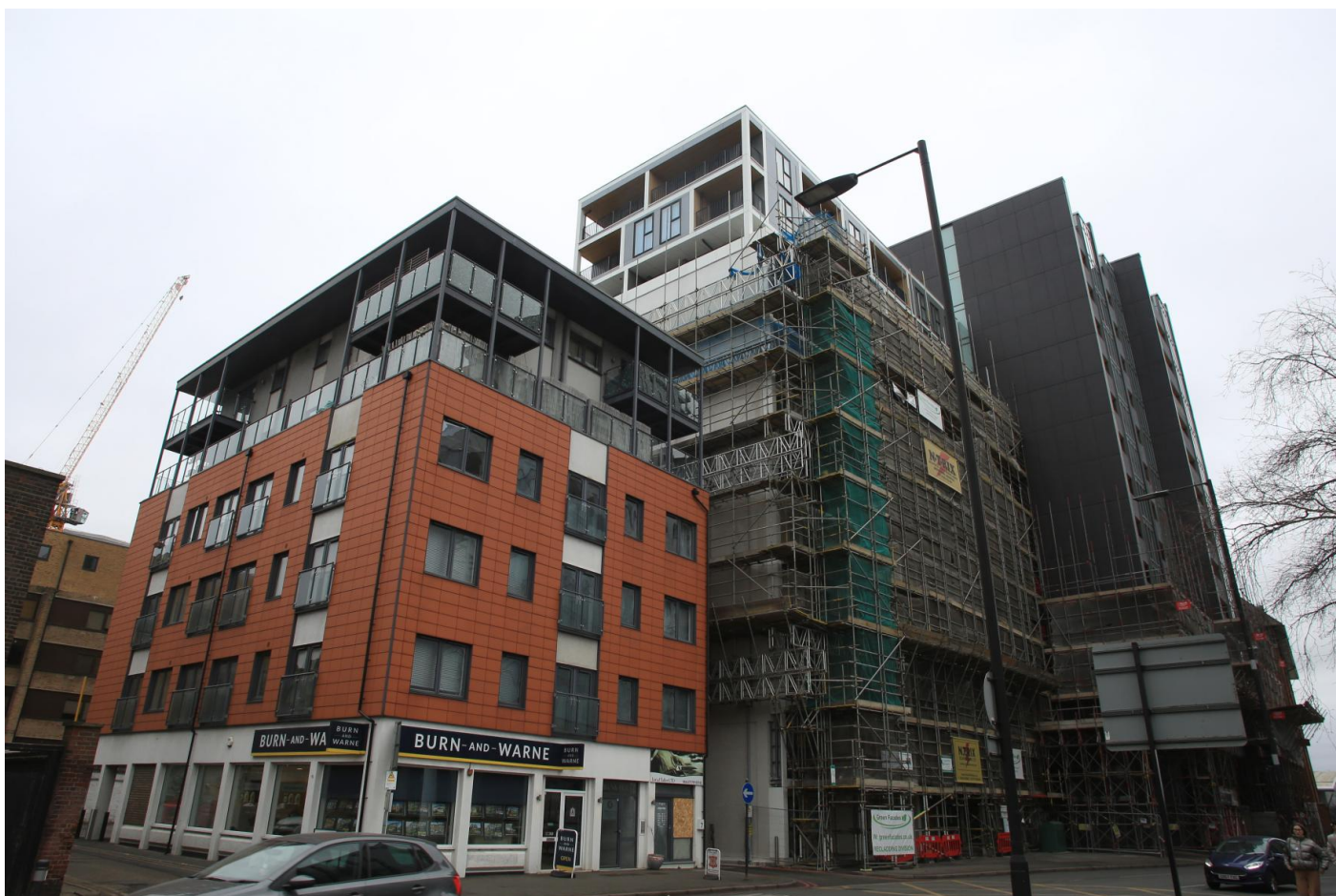
The converted office building in Sutton (with scaffolding) where the couple live PETER TARRY
