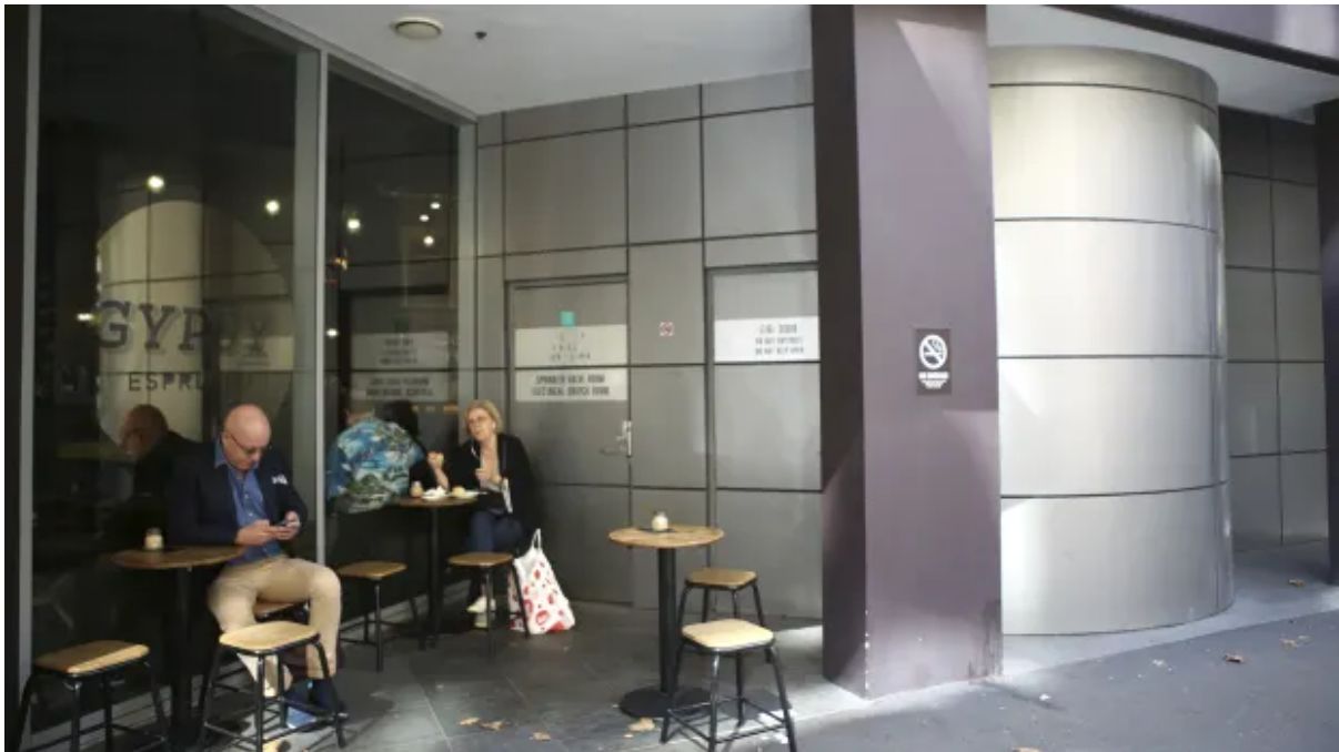
Combustible cladding around ground floor entrances of Sydney's Ikon building will also be replaced under the proposed fix. James Alcock
