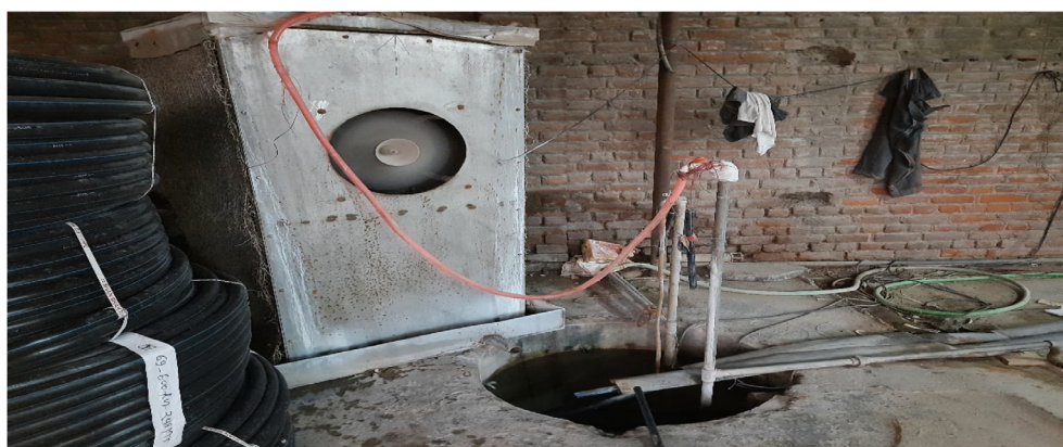
Fig. 4. Water Tank with Cooling Arrangement (New).
