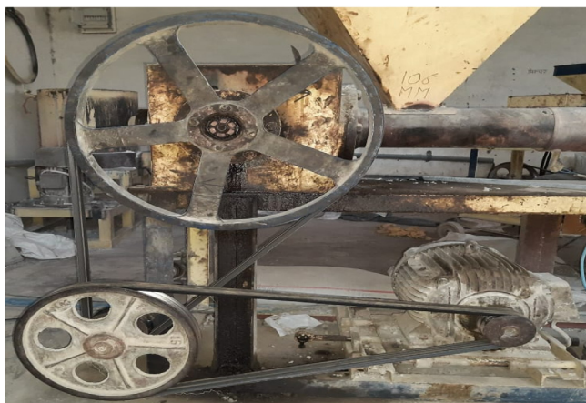
Fig. 7. Pulley Motor Arrangement (Old) Arrangements.
