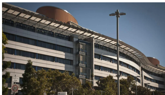
Cladding was removed from the facade of the Princess Alexandra Hospital. Picture: AAP Image/Robert Shakespeare
