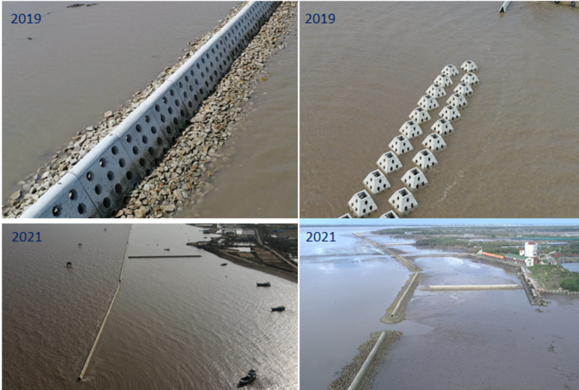
Figure 14. The Hollow Triangle Breakwater constructed in Con Cong, Tan Thanh, Tien Giang, in the VMD (Source: SIWRR, 2021)
