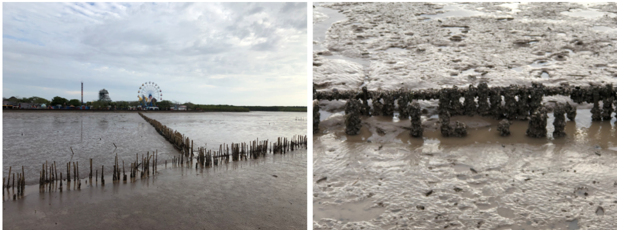
Figure 10. The T-shaped bamboo fence destruction after four years in Nha Mat, Bac Lieu (March 2022) due to harsh environmental conditions and severely corroded by the barnacles (Source: SIWRR, 2022).
