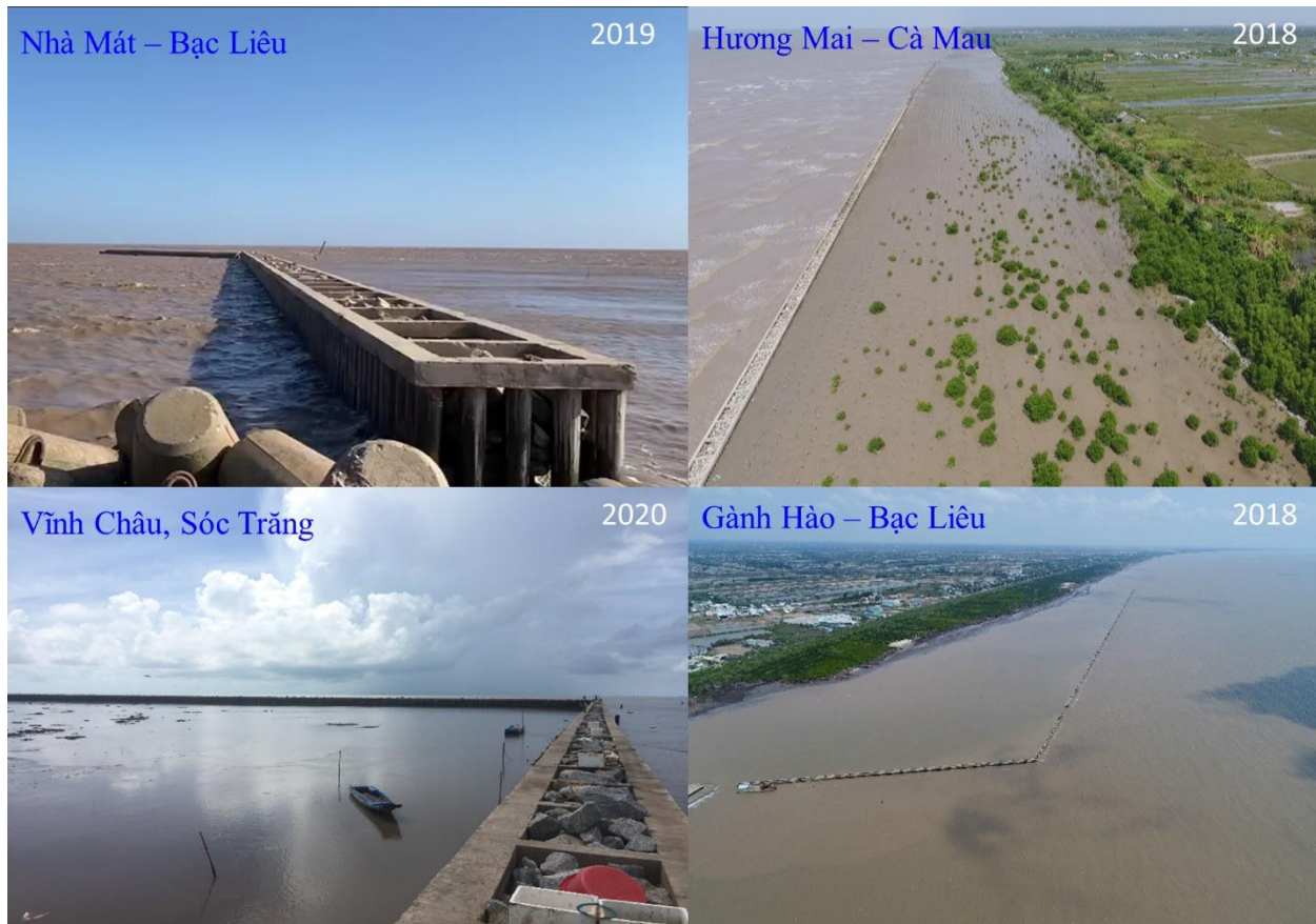
Figure 11. The pile-rock breakwater constructed in Soc Trang, Bac Lieu, and Ca Mau (Source: SIWRR, 2020)
