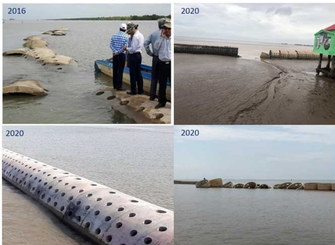
Figure 13. Semi-Circular breakwater was constructed in Nha Mat, Bac Lieu, and Ca Mau. The uneven subsidence of this structure is shown in April 2020 (Source: SIWRR, 2020)
