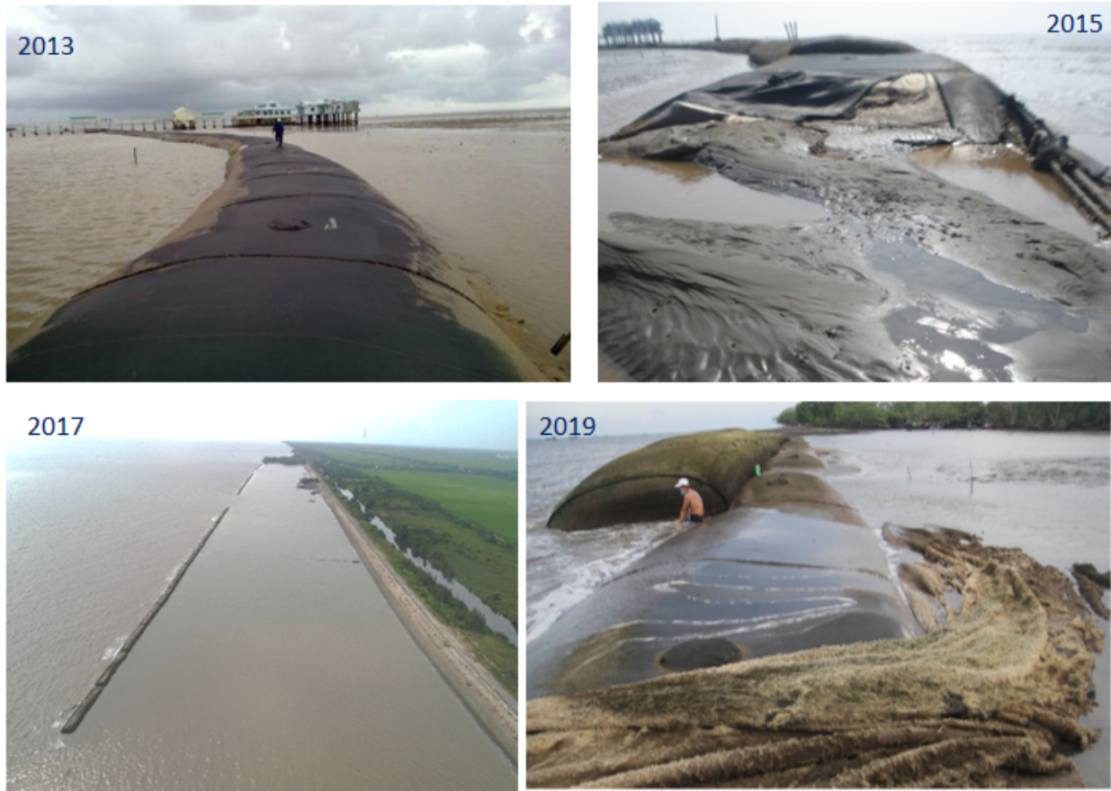
Figure 8. The Geotube breakwater constructed in Nha Mat- Bac Lieu (top panel) and Go Cong Dong and Tien Giang (bottom panel) (Source: SIWRR, 2020)
