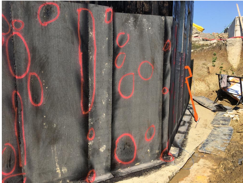
Bitumen liner - poor installation/low quality material
