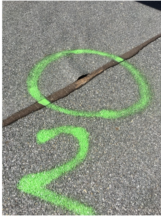
Bitumen liner - poor installation/stress fracture
