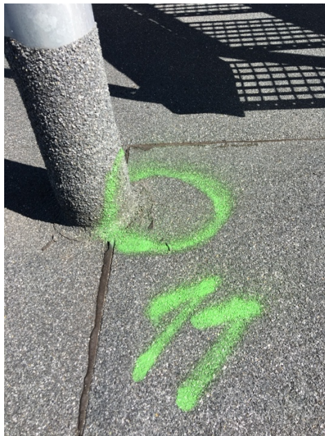
Bitumen liner - poor installation/stress fracture
