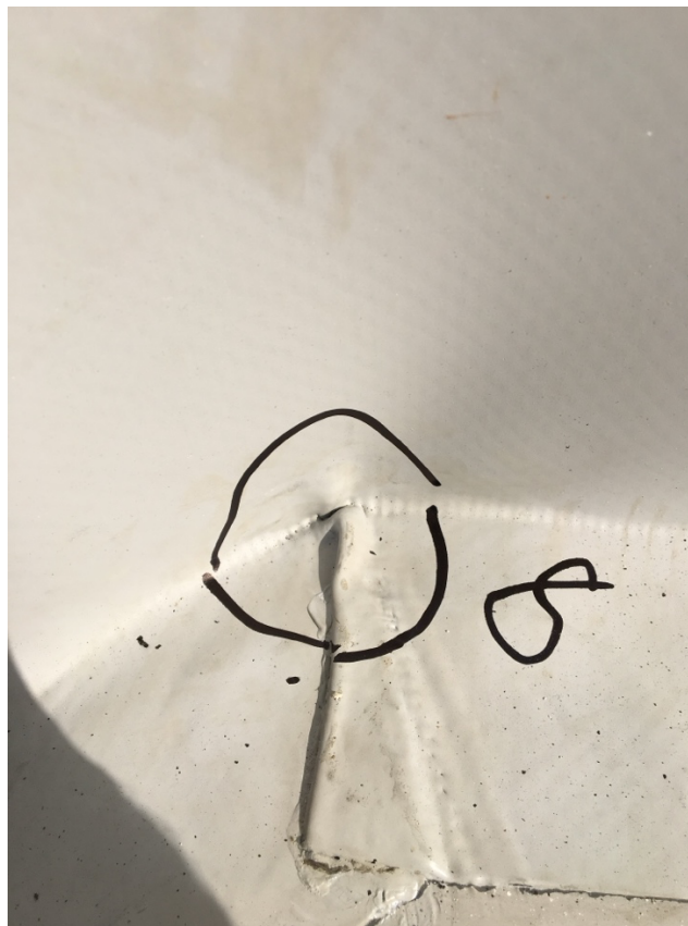
TPO liner - poor welding/stress fracture
