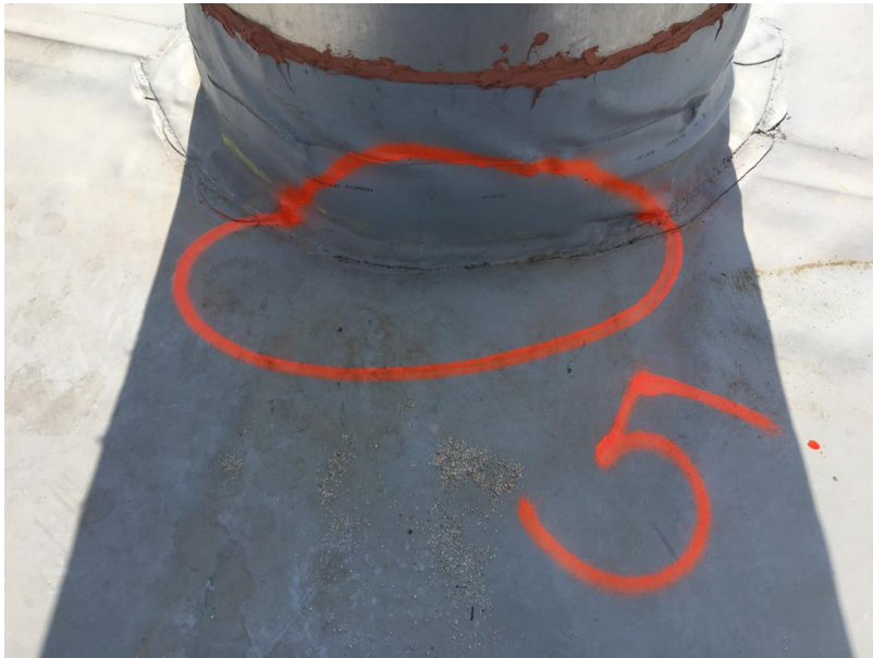
PVC liner - poor welding
