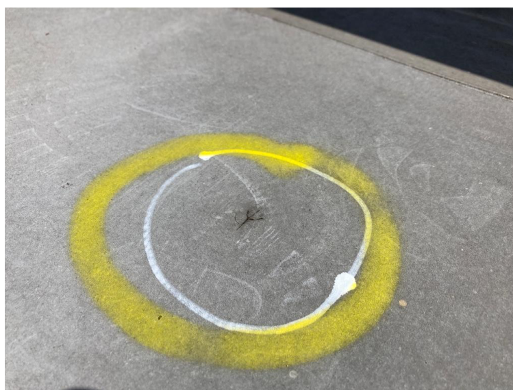
PVC liner mechanical damage – likely caused by a subcontractor or liner installer
