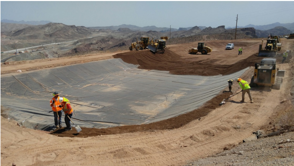
Figure 4: Photograph of 60 mil EIA geomembrane for a secondary containment application with a soil cover.
