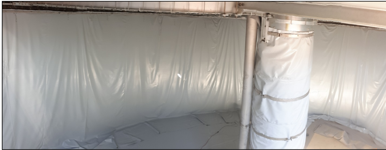
Figure 3: Photograph of grey 45-mil reinforced EIA geomembrane used to re-line and rehabilitate a concrete storage tank for potable water.
