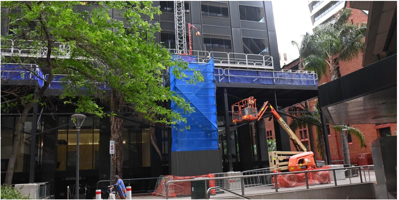
Work has commenced on a replacement of cladding material on the Grenfell Centre office tower. Picture: Keryn Stevens
