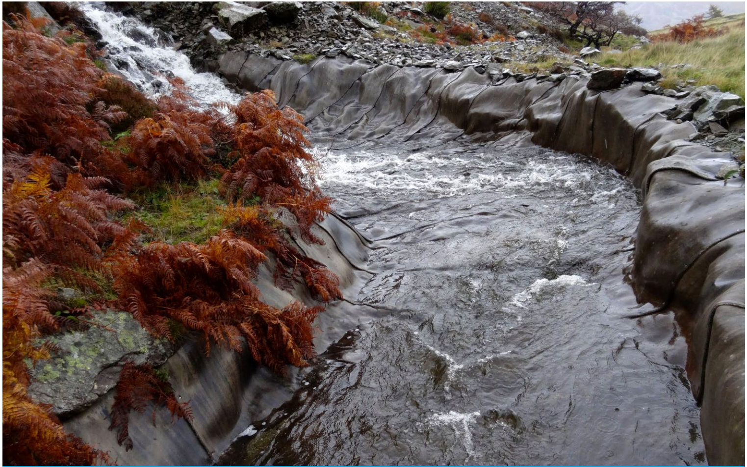
The installation five years later - with an average rainfall of over 2500mm per year, 400mm fell in just six days at the end of October 2021.
