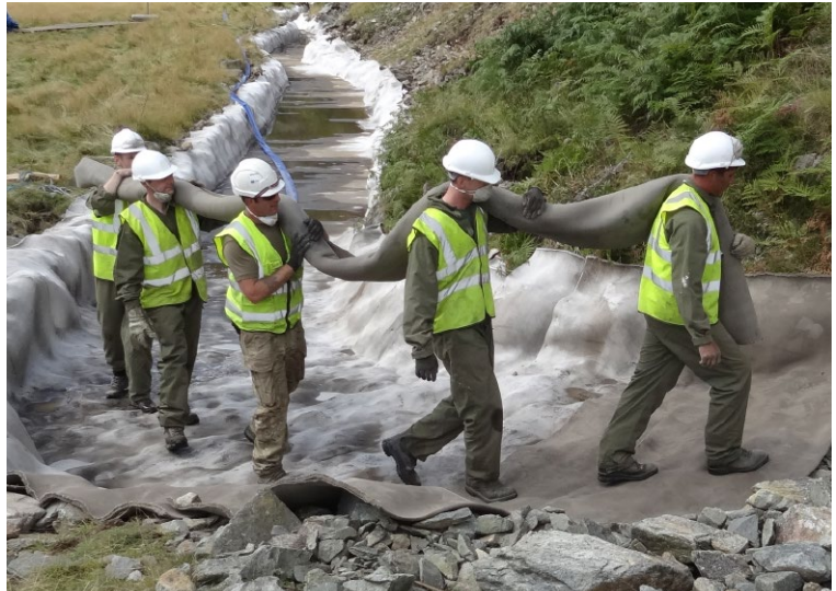
The site was extremely difficult to access, all work was carried out by hand
