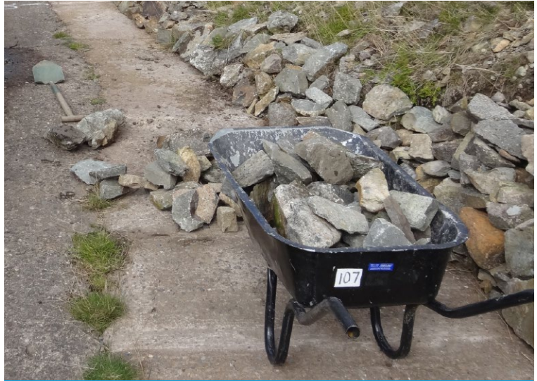
Large stones and debris were cleared to be re-used after CC installation
