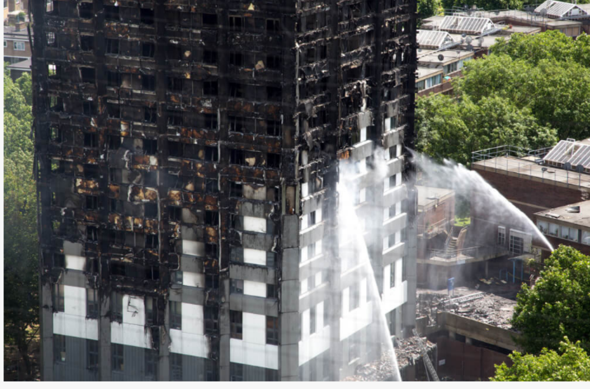
The June 2017 fire that ripped through the 24-storey Grenfell Tower in London resulted in 72 deaths and left many homeless.
