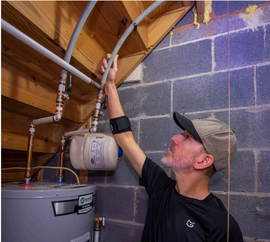
Andrew Boyer shows the Quest pipes that are connected to the water heater in his Ephrata Borough home Thursday, Sept. 12, 2024.
