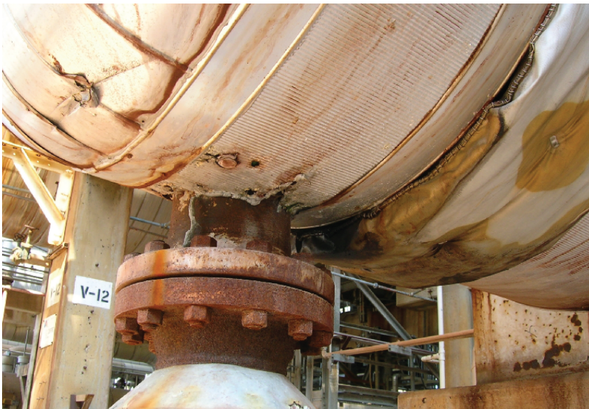
Fig. 4: Plant environment and acidic product leakage have eaten away the aluminum jacketing on this vessel—a clear indicator of moisture-saturated insulation.
