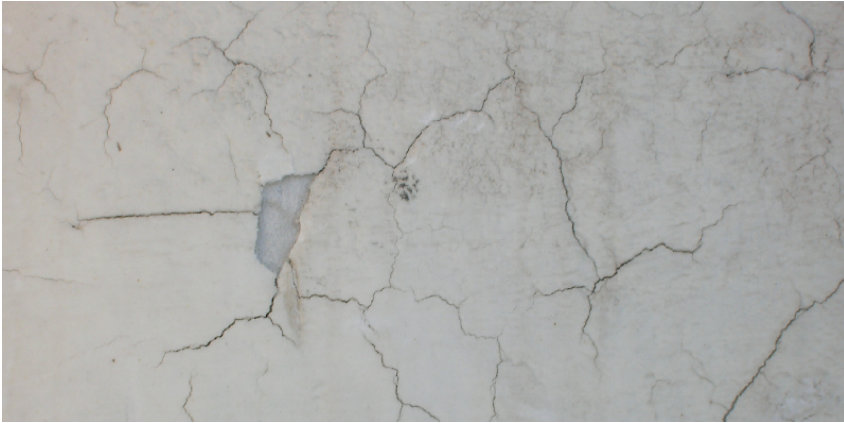
Fig. 2: This acrylic-spray-on insulation failed after two years from excessive film thickness or insufficient dry time between coats during application. The vessel may also have operated at temperatures beyond the acrylic resin's tolerance.
