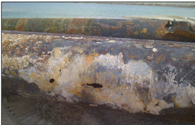
Figure 6: External corrosion in DI Pipes, High
