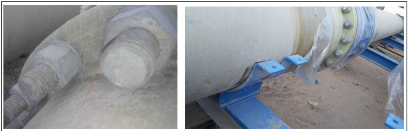
Figure 20: Flange crack, the valve is not supported
