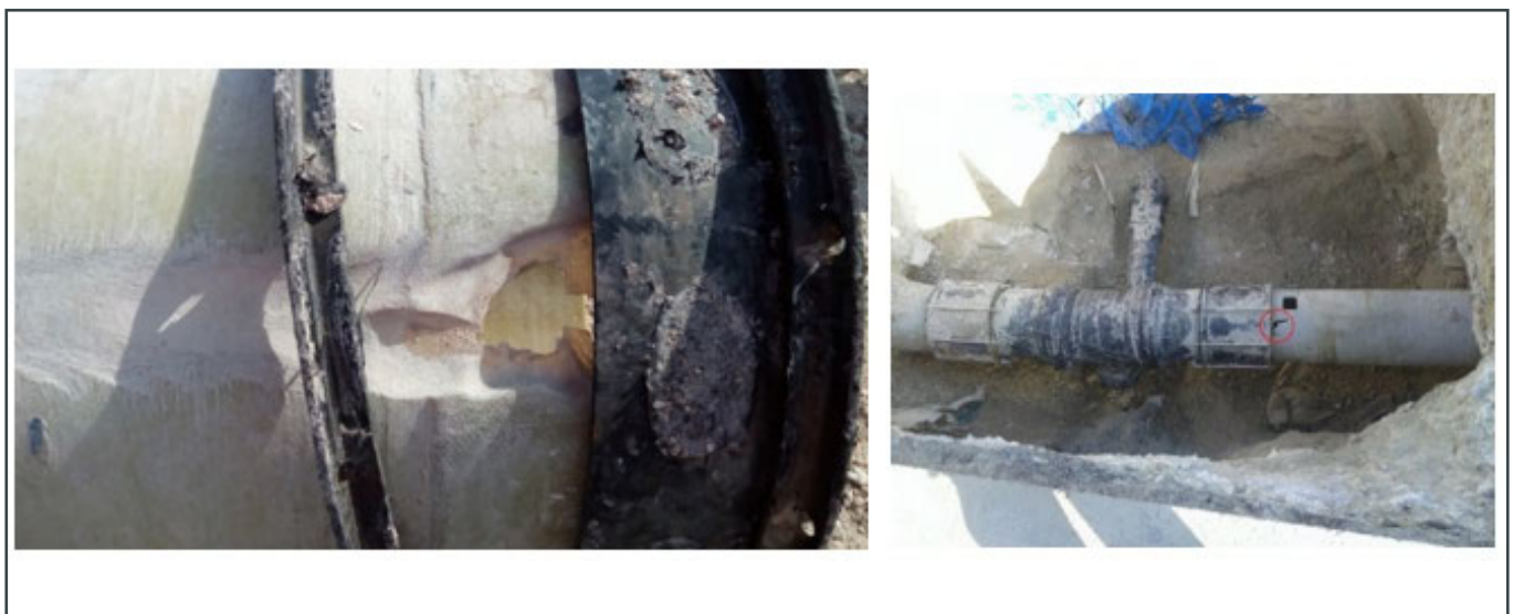
Figure 25: Failure near mechanical coupling
