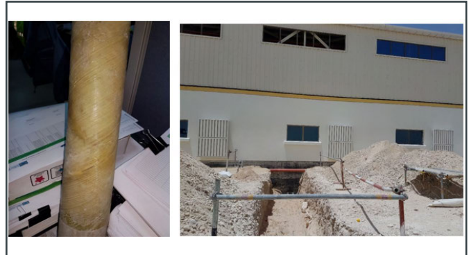
Figure 23: GRE pipe damage due to settlement
