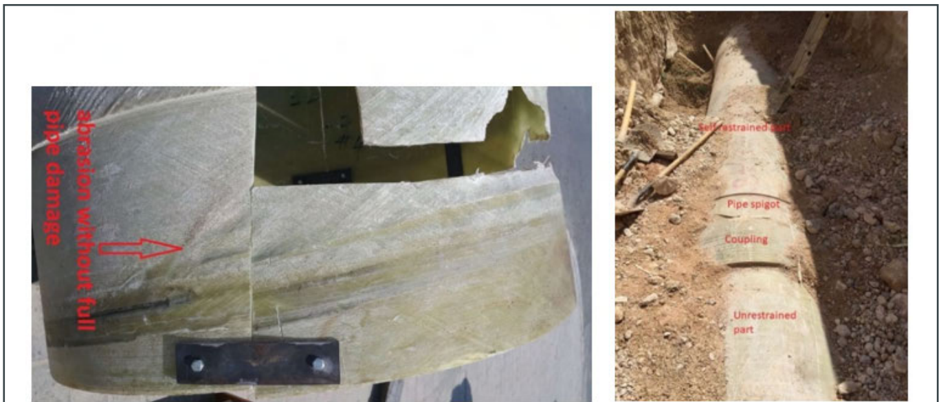
Figure 24: GRP Coupling failure (abrasion on pipe surface)
