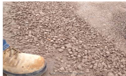
Figure 12. Unacceptable sub grade for direct (HDPE) geomembrane installation [Scheirs]
