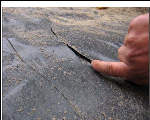
Figure 28. Close up brittle crack in the 45 year old 0.4 mm geomembrane, causing water inflow [Witteveen+Bos / Kiwa, 2010]
