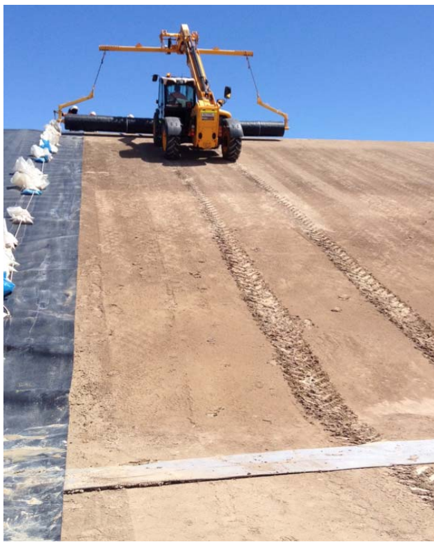
Figure 11. Unacceptable damage to sub grade and improper working method by construction equipment [Scheirs]
