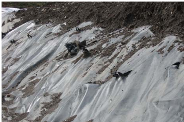
Figure 19. Mechanical damage to a geomembrane anchoring trench by using wrong backfilling equipment (crane) and less instructed personnel on site [Gerritsen]
