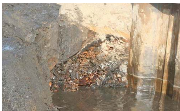
Figure 8. Presence of an un-expected dumpsite with ceramic material and environmental pollutions at a project site with a planned submerged geomembrane [Gerritsen].
