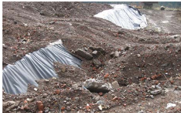
Figure 9. The presence of sharp/big stones without protective geotextiles will significantly increase the risk on damaging the geomembrane [Gerritsen].
