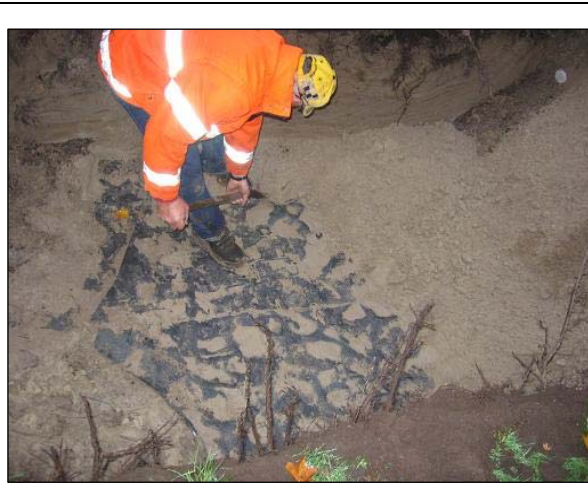
Figure 27. Investigation of 45 year old 0.4 mm geomembrane in trial pit, observing an irregular surface, wrinkles and cracks and water inflow [Witteveen+Bos / Kiwa, 2010]
