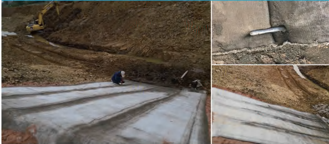
Lake bottom and bank slope of wuhan water park protection project in Hubei province
