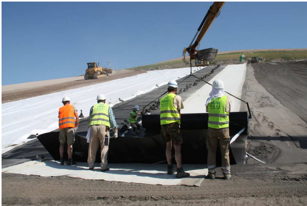
Figure 4: Approved geosynthetics being installed – geomembrane over the GCL and then covered with a geosynthetic drainage mat – on the left placement of cover soil (landfill cap Hanover, Germany)
