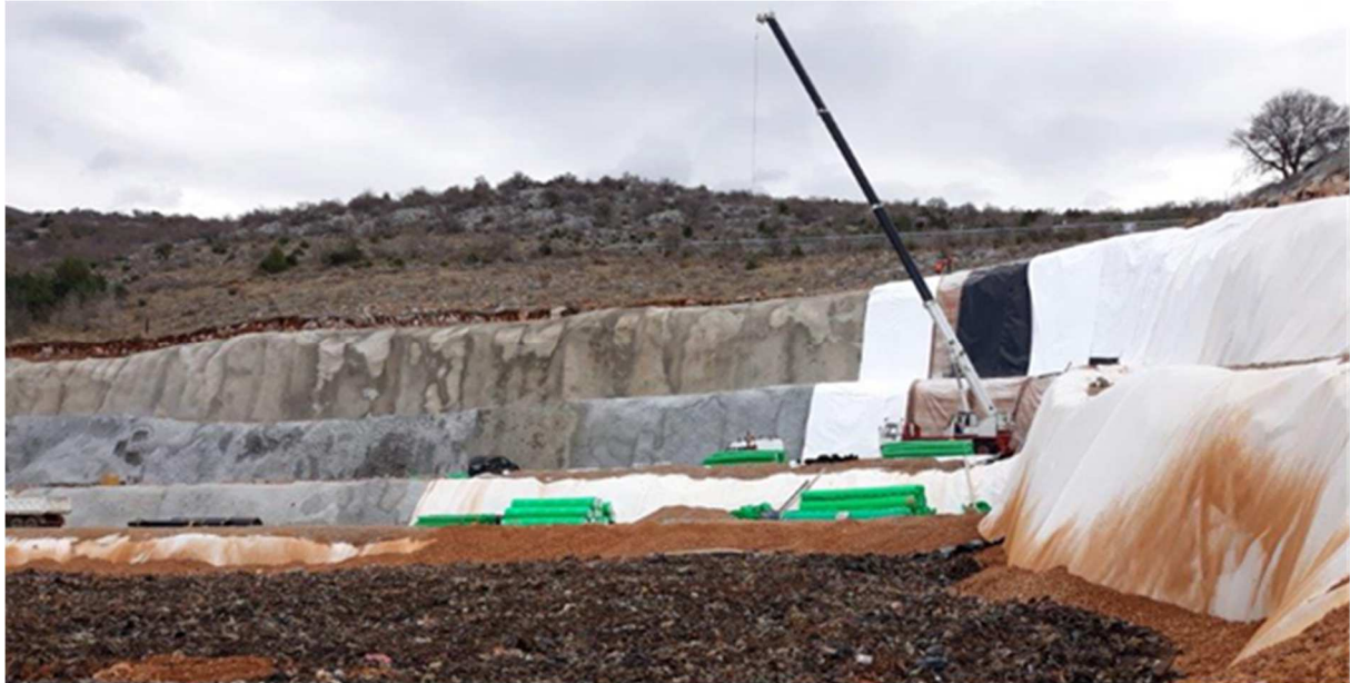
Figure 9: Sealing of the nearly vertical side slopes of the base lining system in the Senj landfill
