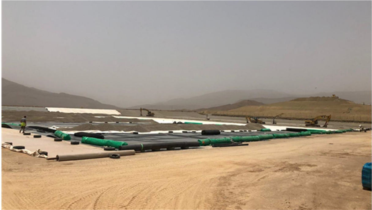
Figure 10: Geosynthetic base lining system with GCL and geomembrane as a composite lining system
