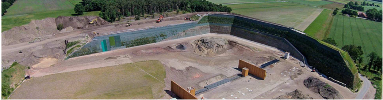
Figure 13: GCL used as an encapsulation barrier for waste construction material in a MSE structure
