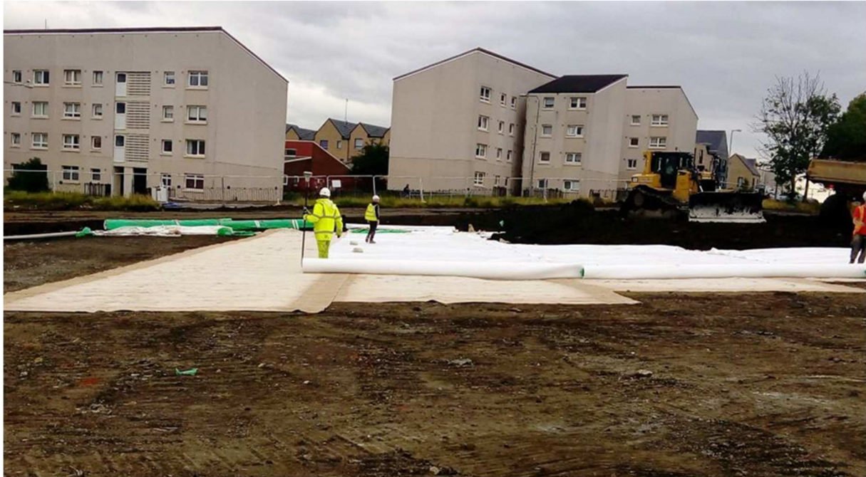
Figure 12: A protection nonwoven geotextile is being installed over a multicomponent GCL and then covered with soil material
