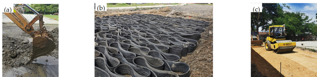
Figure 3. Vehicle platform construction process. (a) Excavation and levelling of the subgrade, (b) placement of the tire geocells, (c) filling and compaction.
