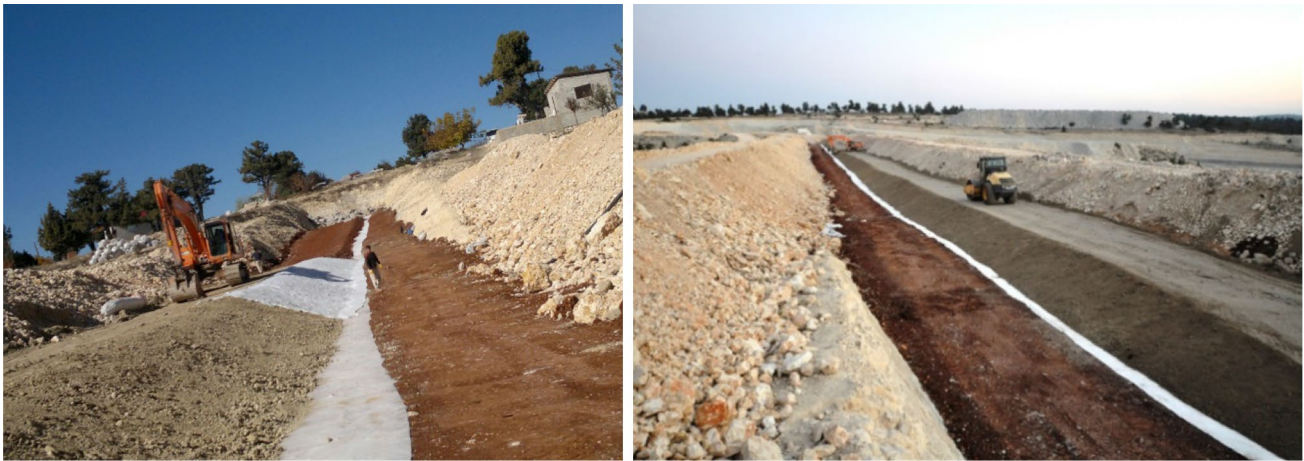
Fig. 17 At left, second stage installation of GLC. At right, placement of the low-quality clay over GCL in Avgadı Dam
