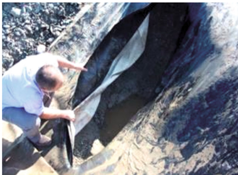
Rupture of the geomembrane on the slope in the area of a pit/track due to poor subgrade preparation
