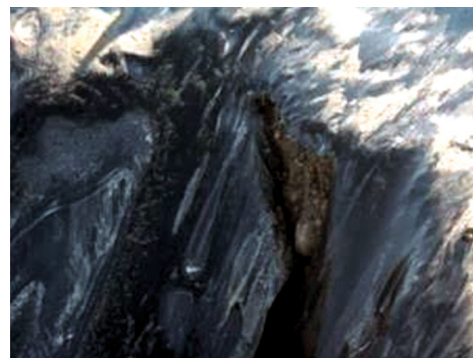
Further expansion of geomembrane rupture in the transverse direction
