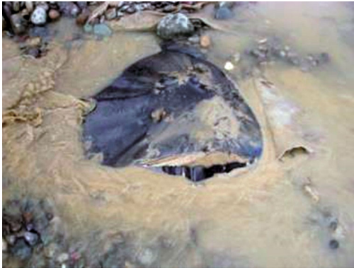
Rupture of the geomembrane along the edges of a boulder embedded in the barrier base
