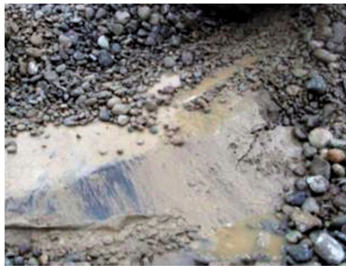
Rupture of the geomembrane along the edges of a sinkhole formed in the sandy-loam bedding at the geomembrane base
