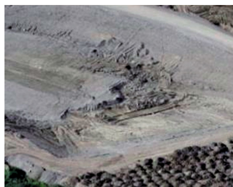
Violation of the subgrade surface by machinery during construction
