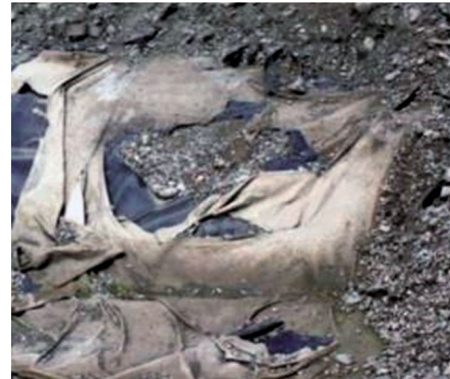
Damage to the geomembrane liner due to its placement on inadequately prepared subgrade
