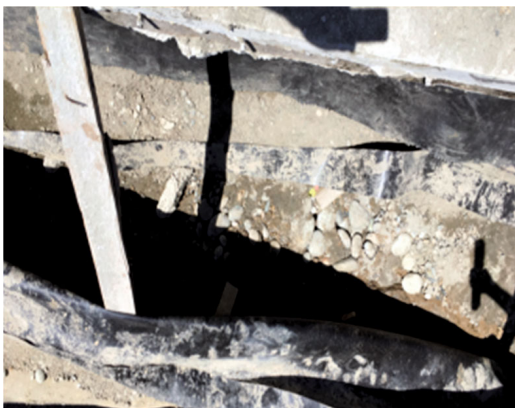
Washed-out cobbles under the breached geomembrane seam
