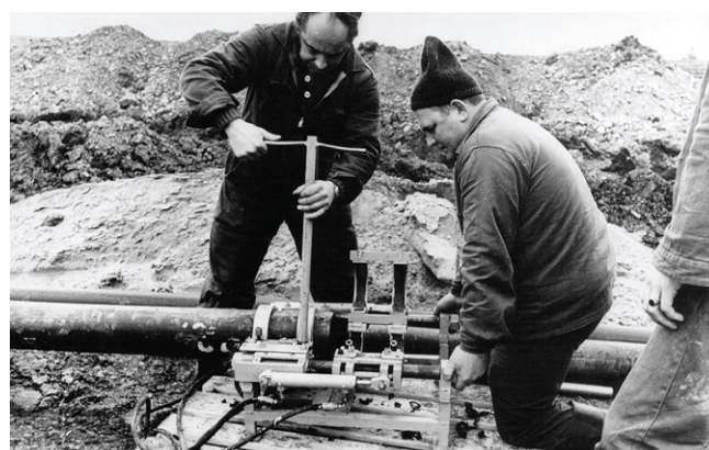
A Polybutene piping installation over 50 years ago
