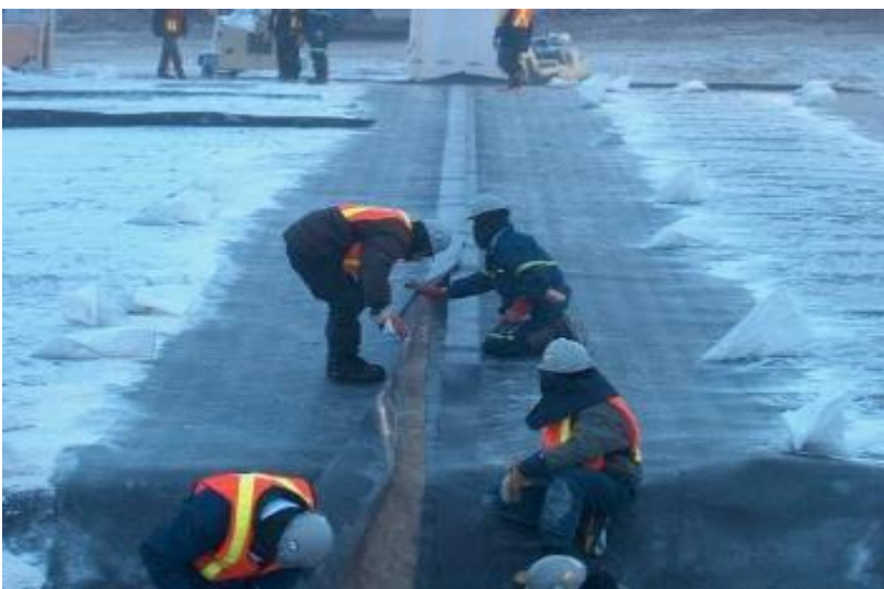
Figure 2.5: Controlling cleanliness of both sides of the geomembrane being welded together (photo courtesy of A&A Technical Services)
