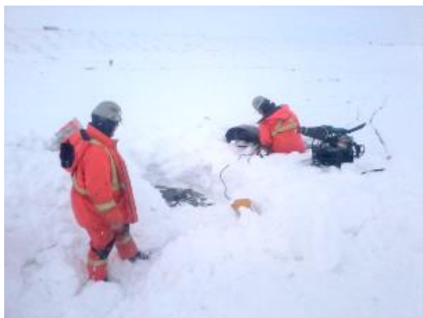
Figure 3.1: Example of GBR covered by a 500 mm snowfall before completing installation (Courtesy FC Geosynthetics)
