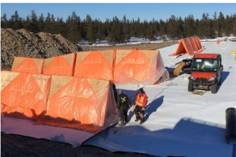
Figure 2.6: Use of tents to control environmental conditions and reduce humidity around a seam (photo courtesy of A&A Technical Services)
