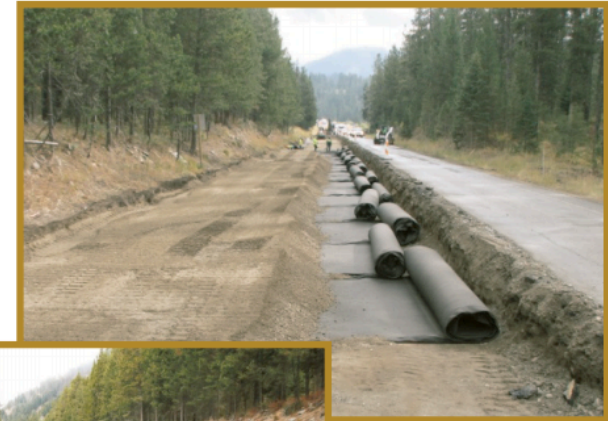
SSDL installed on the northbound lane
