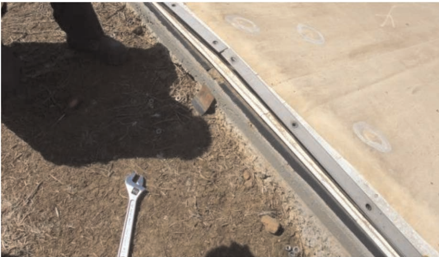
Figure 2. A small liner material sample taken from under a batten bar. This floating cover had many small marked holes which had been caused by embers from a grass fire.
