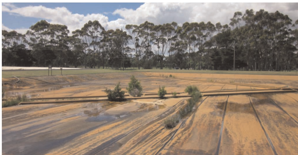
Figure 7. A 30 year old CSPE cover where a lack of maintenance has allowed vegetation to grow.
