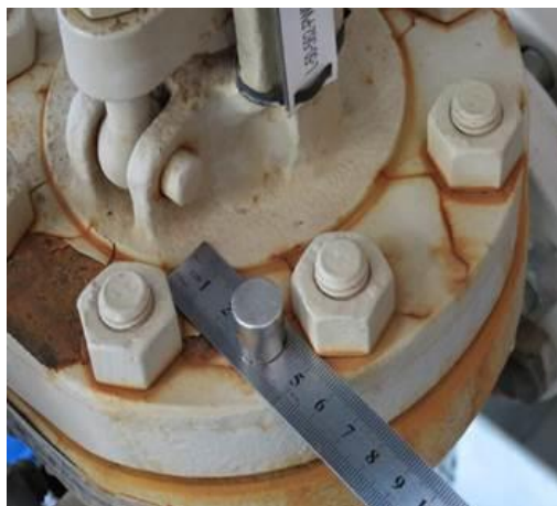
Figure 1: Epoxy phenolic stress cracking around bolted areas
