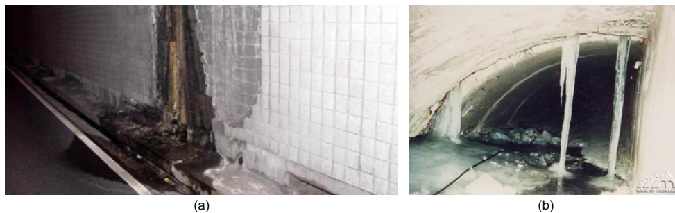
Figure 5. Photo of damaged tunnel lining due to water pressure: (a) photo 1; (b) photo 2
