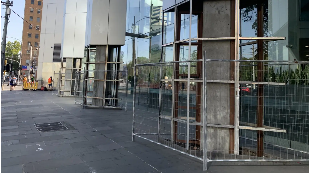
Works under way last month to replace the flammable cladding on the planning department's building at 8 Nicholson Street, East Melbourne.
