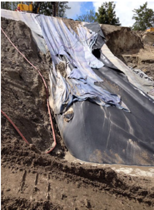
Figure 1 - Slope failure by stability problems after finishing the geomembranes caused by external water pressures versus insufficient backfill levels [Genap]
