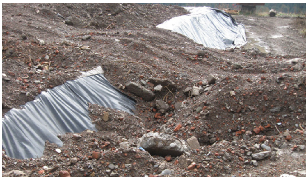
Figure 4 - The presence of sharp/big stones without protective geotextiles will significantly increase the risk on damaging the geomembrane [Gerritsen]
