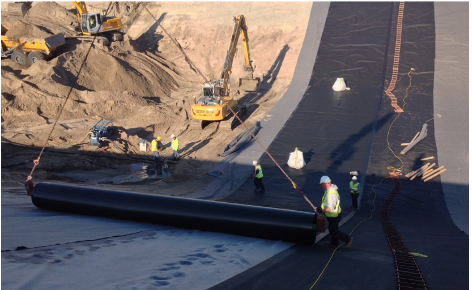
Figure 5 - Example of proper installation using a protective non-woven geotextile at the subsoil and topside of the geomembrane, working sequence with excavation works and installing method at large slopes [Gerritsen]
