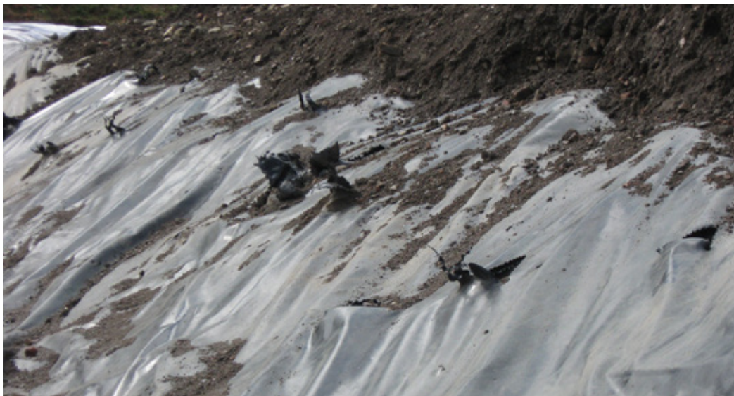
Figure 7 - Mechanical damage to a geomembrane anchoring trench by using wrong backfilling equipment (crane) and less instructed personnel on site [Gerritsen]
