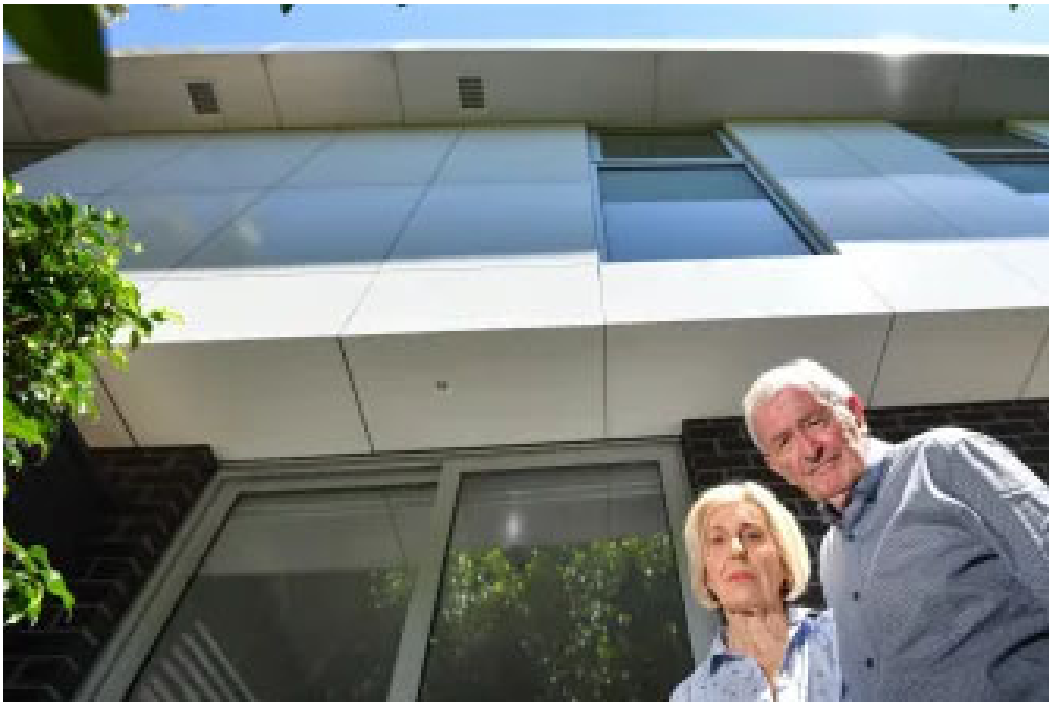
Cladding rectification work at this Williams Road, South Yarra apartment block cost owners $80,000 each according to Jennifer and Kevin Opie. JOE ARMAO
