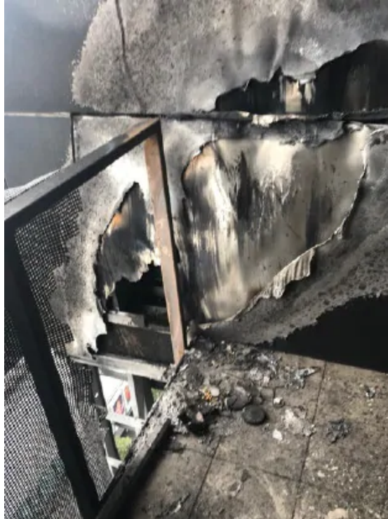
📷 The balcony on the 26th floor of Neo200 building on Spencer Street. Picture: Metropolitan Fire Brigade
