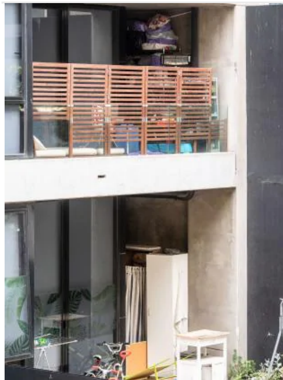
📷 Balconies cluttered with combustible materials and airconditioners covered at Neo200 fire building. Picture: Jason Edwards
