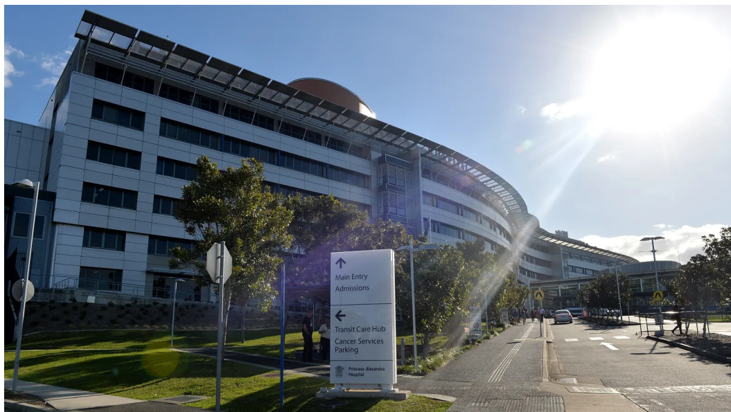
A total of 24 government buildings have been found to feature combustible external cladding. The Princess Alexandra Hospital was among the first in 2017. BRADLEY KANARIS
