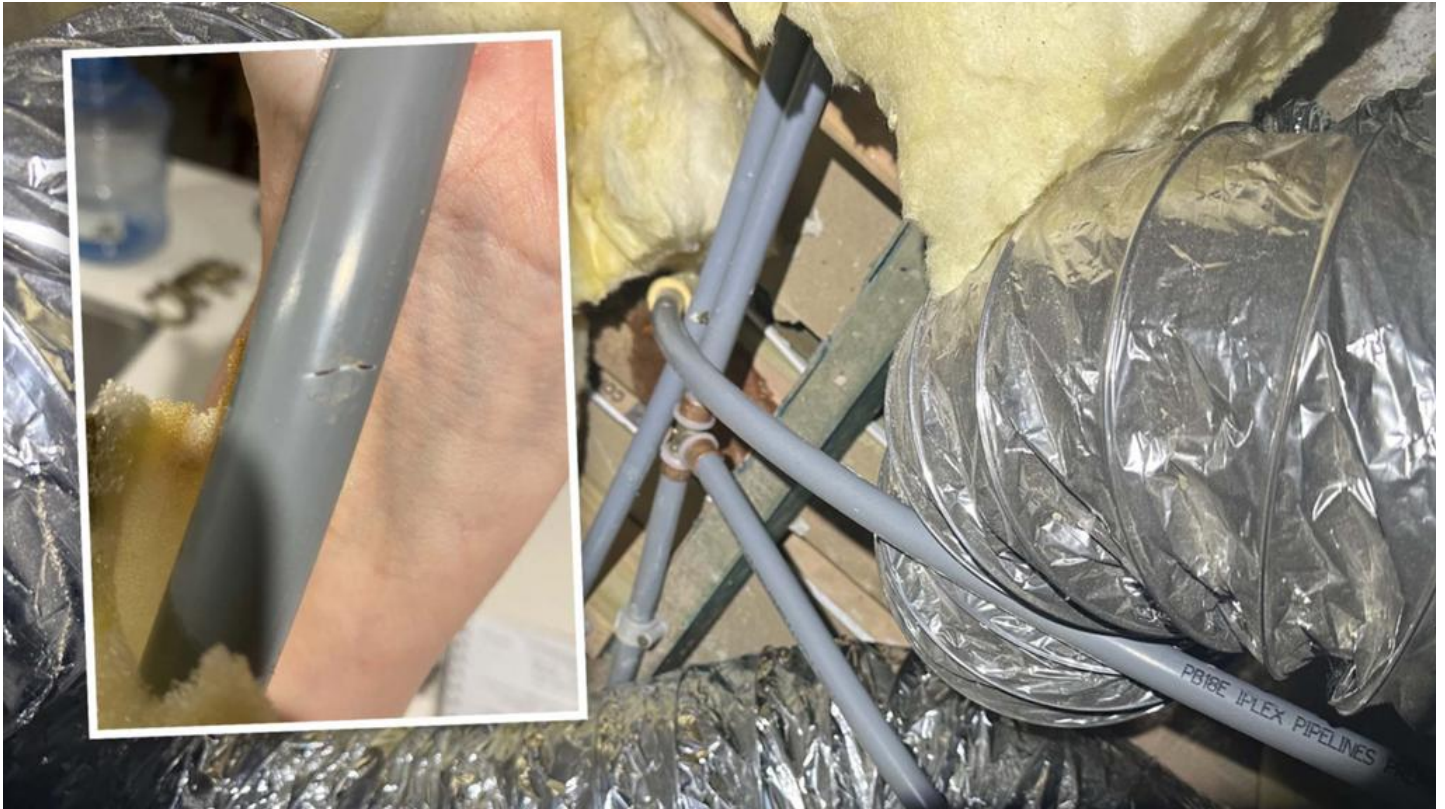
The disputed pipes are installed in nearly 1200 WA households. Credit: The West Australian
